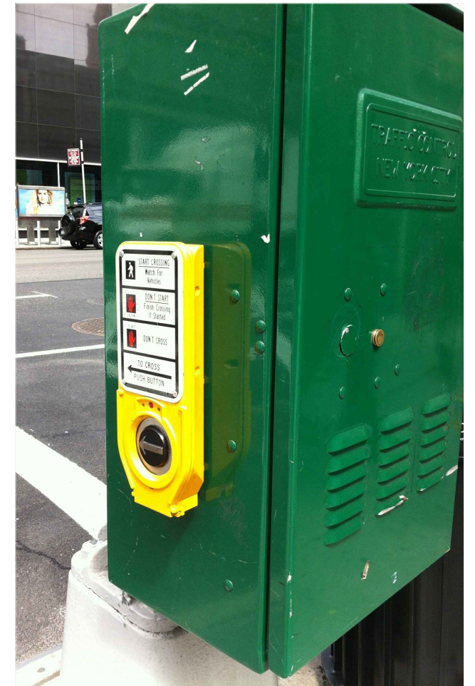
APS ON CONTROLLER CABINER
