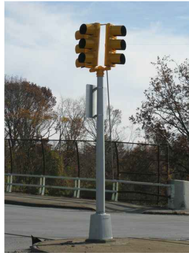
TRAFFIC SIGNAL ON "S-1a" POLE
