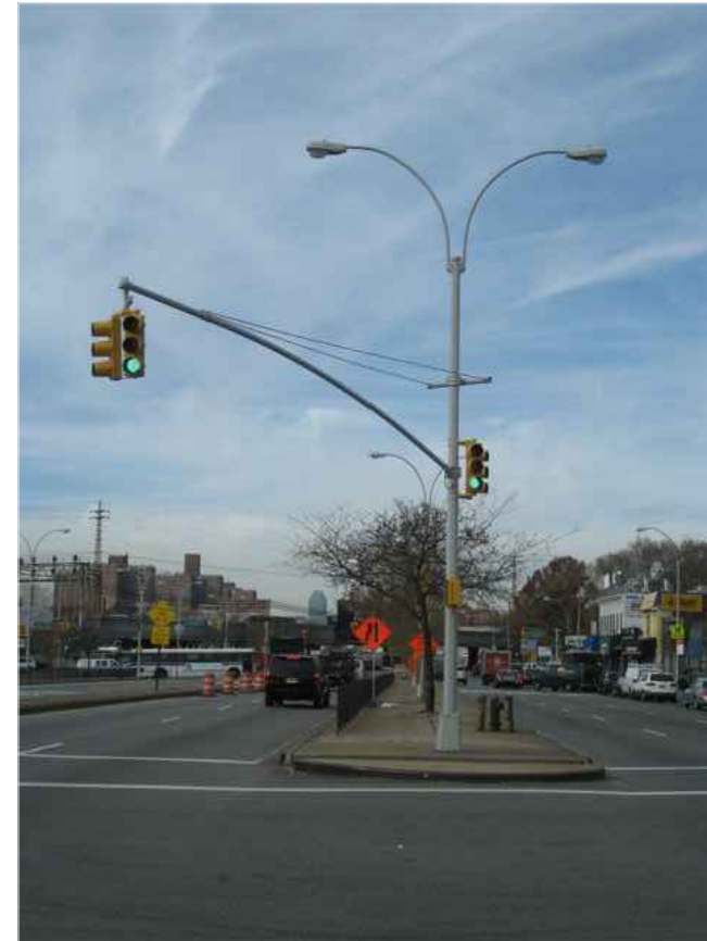
TRAFFIC SIGNAL ON "M-2A" COMBO POLE WITH 180° TWIN ARM TYPE 7" SHAFT EXTENSION
