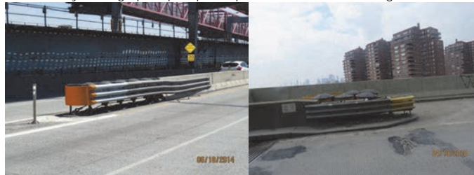
Williamsburg Bridge Impact Attenuators in 2014 and 2018.
