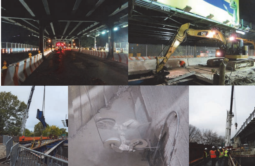
Night Work in August 2017. Stage 1 Deck Demolition in September. Stage 1 Steel Demolition Girder Removal in November 2017. December 2017 - Stage 1C Wire Saw Cutting at The West Abutment. Lifting Out the Cut Pieces.
