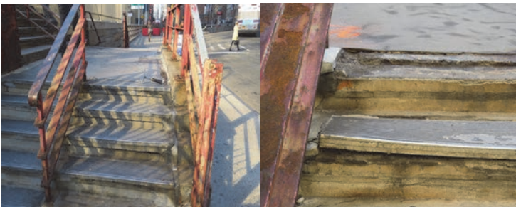
Morris Street Pedestrian Bridge in February 2017: Span #1, Near Beginning Abutment – First Step Tread Plate Missing and Second Tread Plate Broken.
