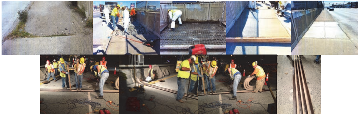
July 2013 Safety Flag: Ironworker and Mason Crews Repairing Missing Joint Seal Materials on the Brooklyn-Bound Williamsburg Bridge. The Joint Sealer Spaces Were Widened on Each Part of the Joint Utilizing the Shop-Made Jack Expansion Blocks, and Then Completely Cleaned With a Needle Gun to Prepare the Surface to be Rough Contacted With Epoxy Glue. After the Glue was Spread on the Sealer Space Surfaces, the Seal Strip was Installed and Tightened. (Credit: Hany Soliman) October 2017: Tripping Hazard on the Right Sidewalk of the Rockaway Boulevard Bridge over Hook Creek.
