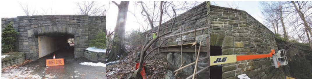
December 2017: Maintenance Workers Adding Mortar to the Joints on the Beginning and Ending Right Side Wing Walls of the Margaret Corbin Drive Bridge over Pedestrian Path Near the North Entrance.
