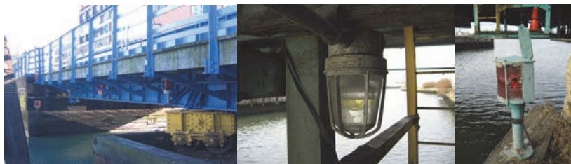
Inspection in Late 2012: Carroll Street Bridge - Navigational Fixtures on North Side of Span – Only the Center Span Fixture was Operational. Grand Street Bridge – Standing Water in the Access Light Fixture at the East Wedge Walkway. Typical Impact Damage to Pier Light.
