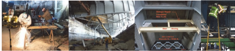
February 2011: Red Flag Stringer Repair at Riverside Drive Viaduct over West 158 th Street. July 2015: Highway Transportation Specialist Andrew Hoang and Assistant Civil Engineer Medina Inspecting a Red Flag on the Manhattan Bridge From the Motorized Bridge Inspection Traveler Platform Beneath the Bridge. (Credit: Tiffany Wong)
