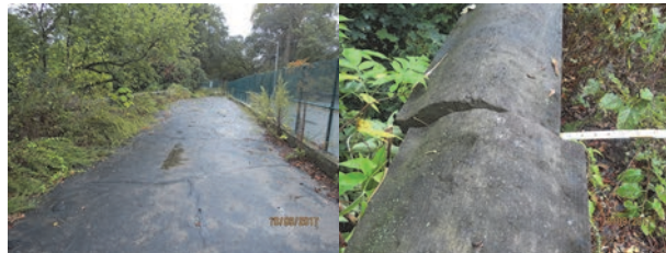
Hill Drive Bridge in 2017: Spans 1 Through 3, Asphalt Wearing Surface - The Deck Top Exhibits Large Areas of Cracked Pavement Due to Deck Deterioration Along the Entire Left Side of the Bridge for a Width of Approximately 12 feet. Most of These Cracks Have Been Sealed With Bituminous Material. Water Seeping Through These Sealed Cracks is Causing Heavy Deterioration of the Deck. Span 1, Stone Coping on Left Railing. (Credit: NYSDOT)
