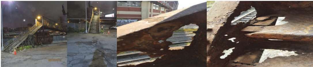
June 2017: Looking North at Spans 3-5, on Left Side - Staircase Stringers and Railing Exhibit Signs of Deteriorating Paint Throughout. End Approach, Looking Northeast – The Approach Wearing Surface Exhibits Spalls and Map Cracks Throughout. September 2017: Close-up View of Holes in Left Side Stringer, Steps and Risers.
