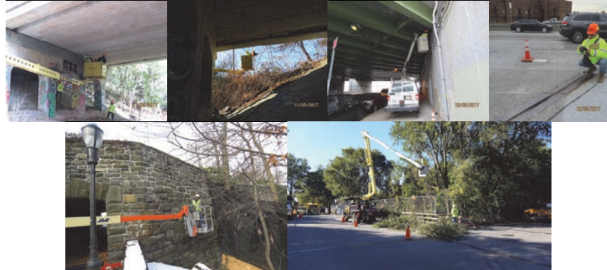
2017: Inspecting Van Name Avenue and Granite Avenue Bridges over B&O Railroad (Abandoned) in November, and Long Island Expressway over Woodhaven Boulevard and Margaret Corbin Drive over Pedestrian Path Near Northern Entrance in December. The Aerial Landscaping Unit of the Agency's Roadway Repair and Maintenance Division Pruning the Trees from the Van Name Avenue Bridge to Enable the Inspection of the Structure.
