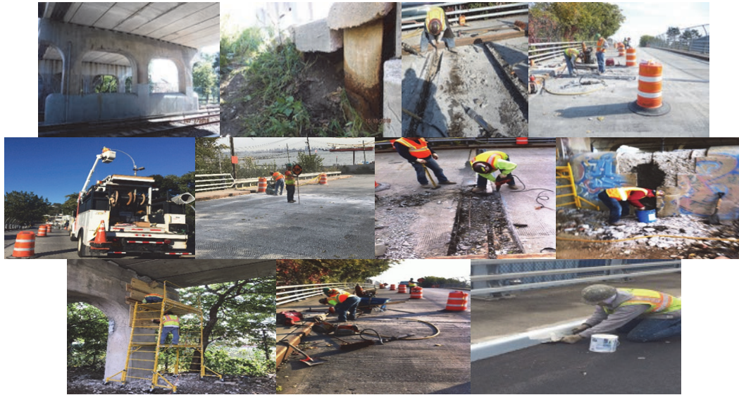
October 2016: Eroded Left Embankment at End Approach. (Credit: NYSDOT) November 2016. During Construction.
