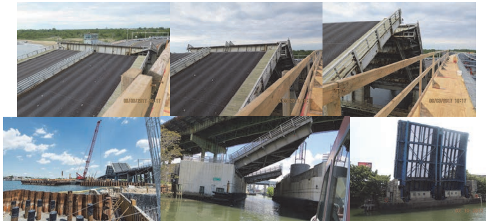
Old Mill Basin Bridge Opening During Construction of the New Bridge in June 2017. Hamilton Avenue Bridge Open in May 2017. Metropolitan Avenue Bridge Over English Kills Open in July 2017. (July Credit: NYSDOT)
