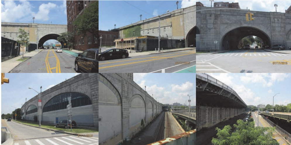
2015: Left Elevation Span 14, Spans 15 – 20. Right Elevation Span 14, Spans 13 – 1, 15 – 77, 41 – 77, and 43 – 13 (Section over NYCDOT Maintenance Garage Area). (Credit: NYSDOT)
