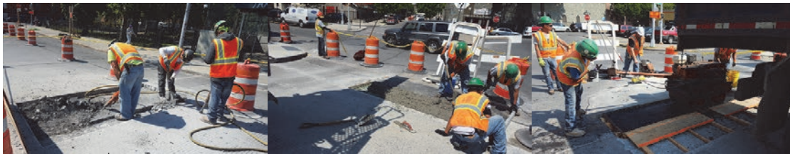
East 162 nd Street Bridge During Construction - Overlay Excavation. Concrete Overlay. Asphalt Placement.
