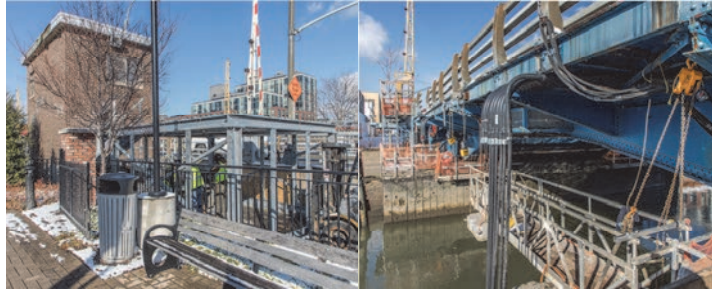
December 2017: Third Street Bridge Generator Platform. Droop Cables.
