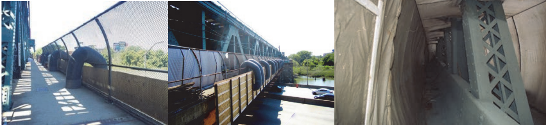
September 2016: - The Contractor Employs a Vacuum System to Capture Lead Particles During the Lead-Abatement Process. This is Done Using Negative Air Pressure to Prevent Emissions From the Abrasive Blasting Process Used to Remove Lead Paint. All Blasting is Done Within Negative Air Containment Units to Protect the Public From Emissions. View Inside the Containment – Bascule Span, Looking East.
