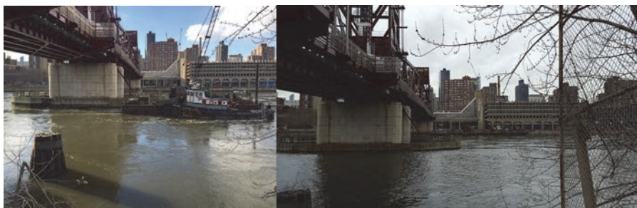
2017: Timber Fender Wall Repairs at the Roosevelt Island Bridge. (Credit: Thomas Leung)
