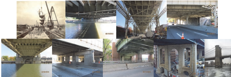
Madison Avenue Bridge Center Pier Under Construction in September 1909, Pier 2 of Broadway Bridge Piers 12, 33, 37, and 42 of Macombs Dam Bridge. (Credit: NYSDOT) Pier 1 (Looking East) of Hutchinson River Parkway Bridge over Hutchinson River. Pier 6 of Manhattan Bridge. Pier 39 of Brooklyn Bridge. (Manhattan and Brooklyn Bridge Credit: NYSDOT)
