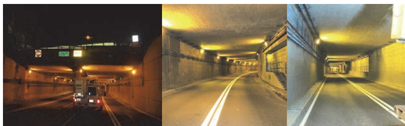
Battery Park Underpass - September 2013 - Span 2 Looking Westbound (FDR Drive to West Street). June 2014 – The Underside of the Tunnel is Completely Covered With Tiles.
