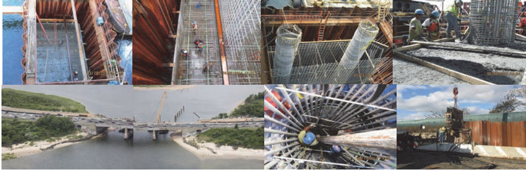
Gerritsen March 2014: Setting Footing Rebars Prior to Placing Pier Rebars and Concrete at Pier No. 2. April 2014: Setting Rebars for Footing and Pier Inside Cofferdam at Pier #1. May 2014: Plinth and Column Reinforcement Inside the Cofferdam for Pier 2. June 2014: Placing and Vibrating Concrete for Plinth at Pier #1. Rebars for Column in Place. West Abutment of Bridge. New Roadway Under Construction at top Next to Westbound Lanes. East Abutment of Bridge. Crane on Barge at Cofferdam for New Pier #2. August 2014: Workers Inside Rebar Cage During the Pumping Concrete Operation at the Pier #2 Column. November 2014: Steel Sheeting in Place for the East Approach Temporary Access Roadway.
