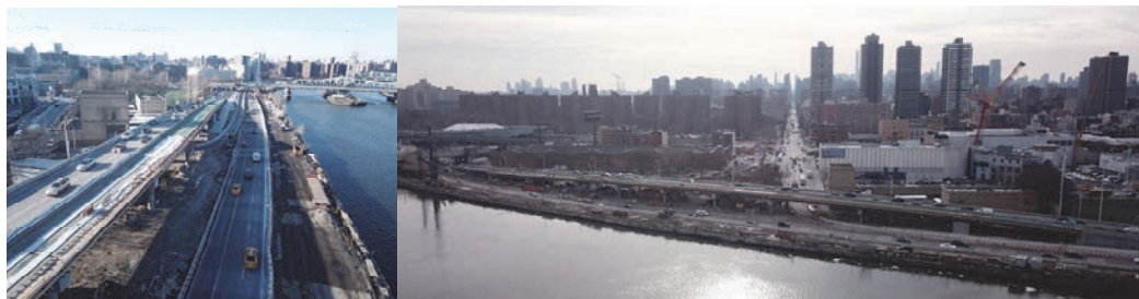
Drone Views: View North Along the Harlem River Drive – the Southbound Bridge Deck is Halfway Constructed. View South Down 2 nd Avenue.
