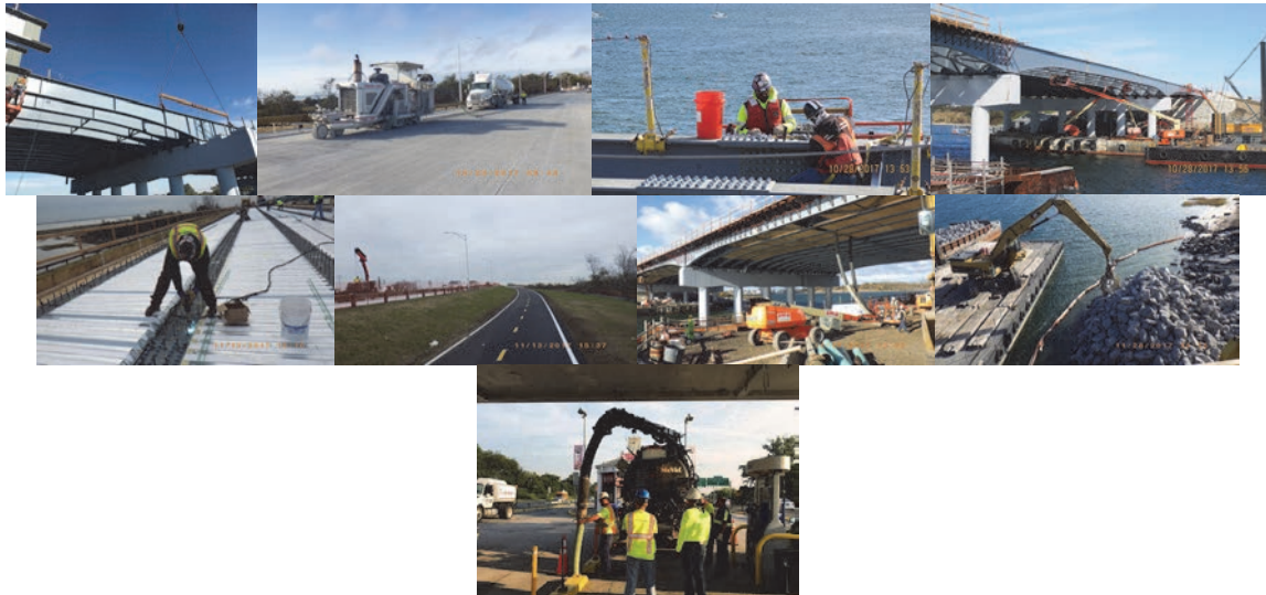
Gerritsen Inlet October 2017: Erecting Final Eastbound Girders at the Gerritsen Inlet Bridge. Pier #1 at Right. Westbound Approach Pavement of the Bridge During Pavement Grinding Operation. Grinder at Left, Water Truck at Right. Working From Man-Lifts on Barges Bolting the Steel Connections. (Manlift Credit: Jessica Wang) November 2017: Welding Shear Stud Connector to Top Flange of the Bridge Girders on the Eastbound Side. Newly Paved Bicycle/Pedestrian Asphalt Path on the Eastbound Side of the Belt Parkway at the West Approach to the Bridge. Pier #2 Facing West, Hot Air Hoses in Place Which were Used to Maintain Curing Temperatures When the Eastbound Deck Concrete was Placed in Late November 2017. Barge-Mounted Crane Placing Riprap Stones on the South Slope of Gerritsen Inlet at the West Abutment. The Turbidity Curtain Prevents Contamination of Jamaica Bay Riprap Placement Will be Completed in Spring 2018. Crew Members Clean out the Drainage Pipe at the Gas Station Near the Bridge to Alleviate Long-Term Flooding Conditions on the Belt Parkway.
