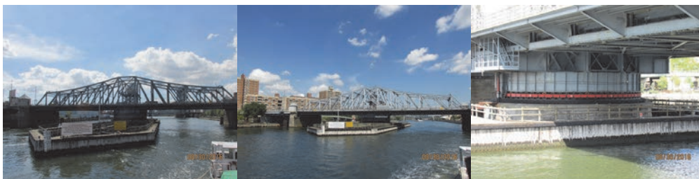
Madison Avenue Bridge in 2016: Left and Right Elevations Spans 12 to 15. Pier 13 – Existing Rack and Pinions. (Credit: NYSDOT)
