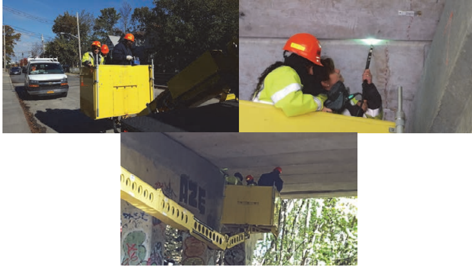
November 2017: Assistant Civil Engineers Sarah Jurado and Nahed Yaaqoub Utilizing a Borescope at the Van Name Avenue Bridge Over B&O Railroad (Abandoned) in Staten Island. The Snooper was Operated by Assistant City Highway Repairer Derrick Butler.
