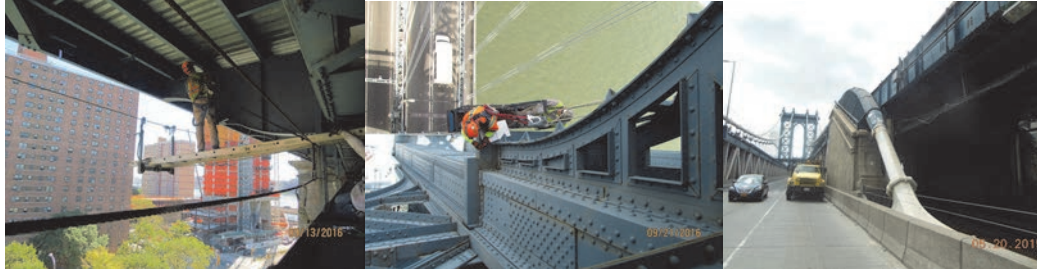
2016: Inspecting the Bridge Using a Scaffold and Sky Climber. (Credit: NYSDOT) Bridge Saddle.
