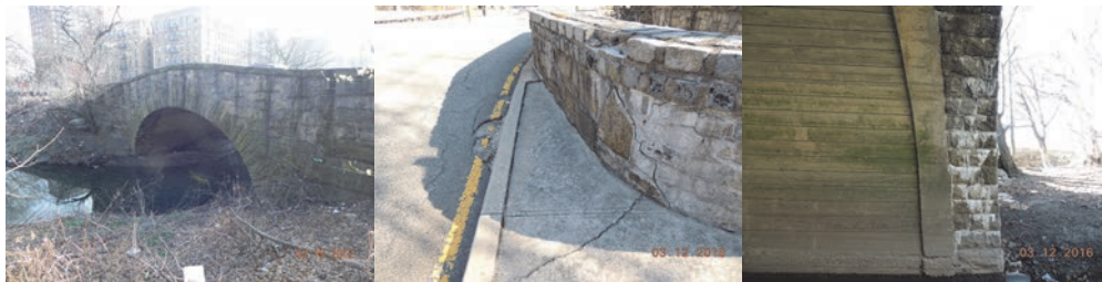
Bronx Boulevard Southbound Bridge Over Bronx River. March 2012: Elevation Left Span. March 2016: Span 1, Right Parapet - Exhibits Spall With a Full Height Vertical Crack. Span 1 – Efflorescence on Underside of Stone Masonry. (Credit: NYSDOT)
