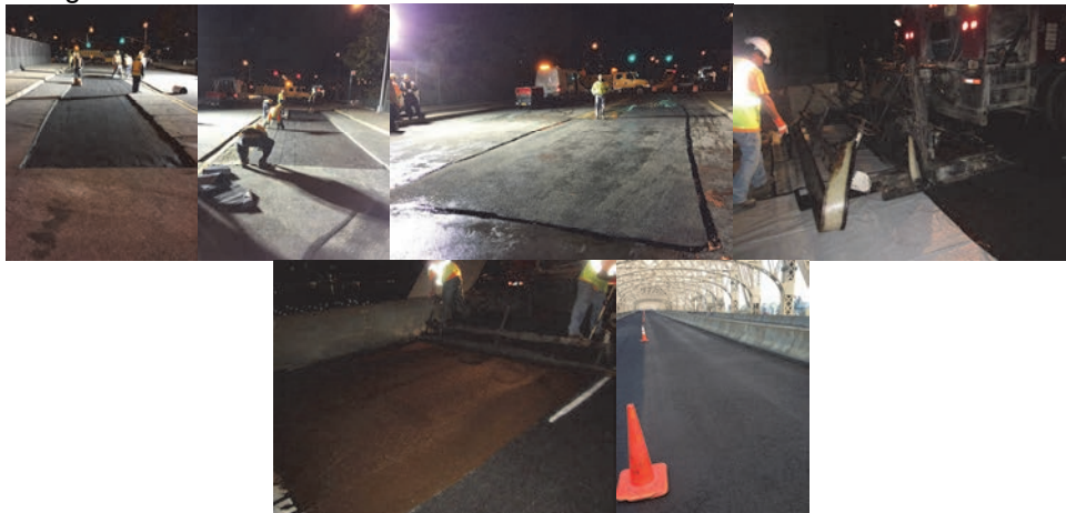
November 2014: Wearing Surface Repairs at 149 th Street over the Cross Island Parkway. Applying the Waterproofing Membrane. The Finished Patch. (Credit: Steve Mezzacappa) Resurfacing the Deck of the Queens-Bound Upper Roadway of the Ed Koch - Queensboro Bridge in June 2014. (Credit: Sunil Desai)
