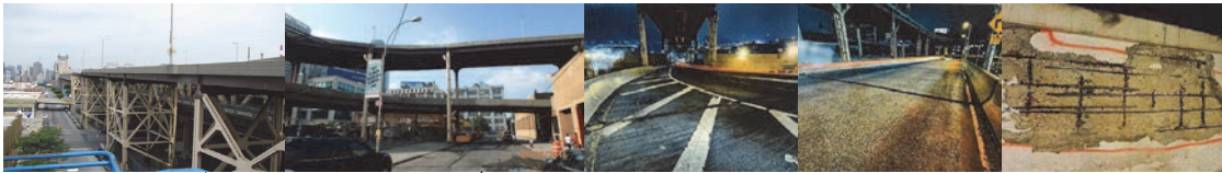
Ramp to 21 st Street From NY Over 22 nd Street. September 2016: Elevation Right Spans 37 to 39. (Credit: NYSDOT) Before Construction.
