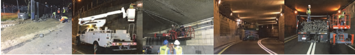
May 2015: Paver Installation in Battery Park. June and July 2015: Removing Existing Conduits at West Street and Battery Park Underpasses. (Credit: Reza Sharif)
