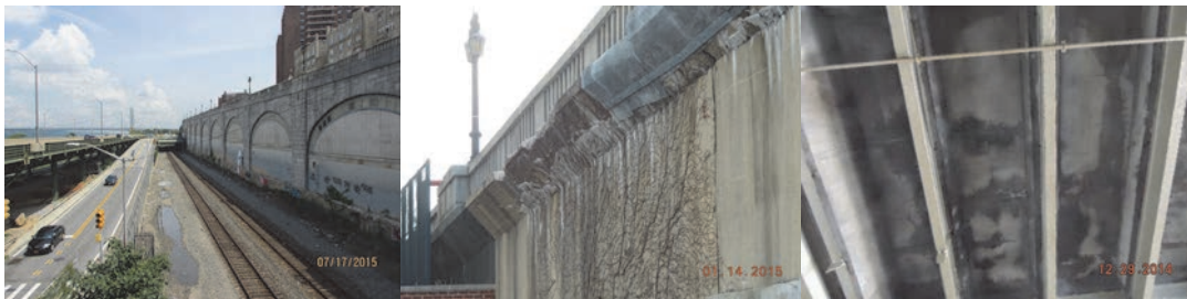
2015: Spans 19-21, East Fascia Overhang, Looking Southwest - Large Edge Spalls with Numerous Cracks and Heavy Efflorescence Throughout Overhang. Span 52 Looking South - General View of Underside of Deck Showing Extensive Dampness and Cracks with Efflorescence.
