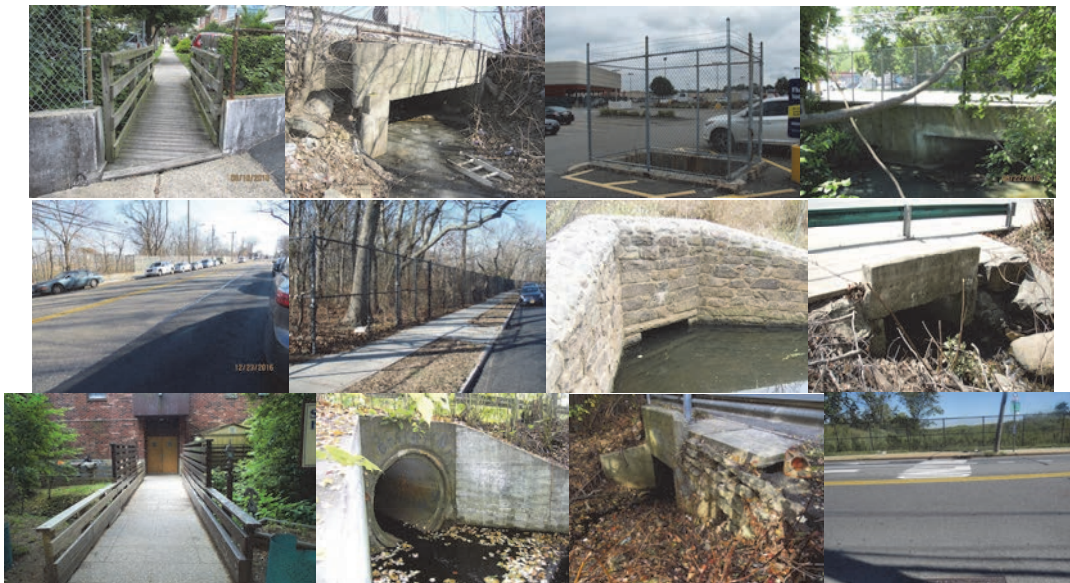
2016: Galloway Avenue over Marianne Street – Wearing Surface, Looking Northwest. Forest Avenue over Crystal Avenue (2 Views). Midland Avenue over Hylan Boulevard (3 Views) – New Asphalt Wearing Surface. Culvert Top – Fence and Sidewalk. Rockland Avenue over Brielle Avenue. Forest Avenue over Randall Avenue. Gregg Place over Randall Avenue. Arthur Kill Road over Muldoon Avenue (2 Views). Arthur Kill Road over Ridgewood Avenue.
