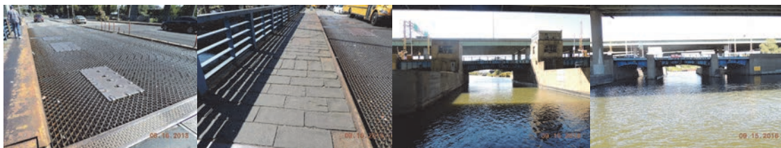
2015: Span #9, Open Deck Grating at Westbound Roadway, Looking Ahead and Right. Loose and Bouncing Plates. Plastic Delineator Posts Mounted to the Concrete Median are Missing the Majority of Posts Due to Vehicular Impacts. Span #9 Right Sidewalk, Looking Back. Asphalt Tiles Over the Bascule Span are Severely Deteriorated and Exhibit Several Missing Tiles. Existing Bridge in September 2016 – Left and Right Elevations. (Credit: NYSDOT)
