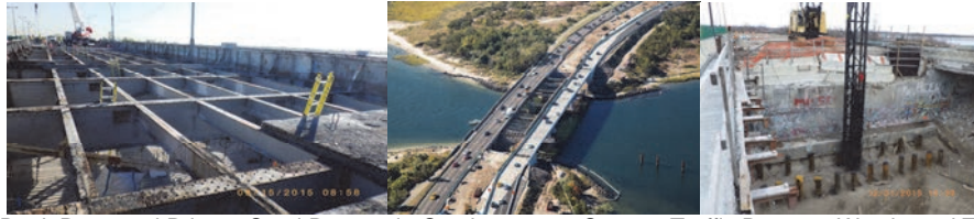
Deck Removed Prior to Steel Removal. October 2015: Stage 2 Traffic Pattern. Westbound Traffic at Right on New Bridge. Eastbound Traffic at Left on Existing Bridge. December 2015: Driving 14-Inch Diameter Steel Shell Piles at East Abutment - Facing East.
