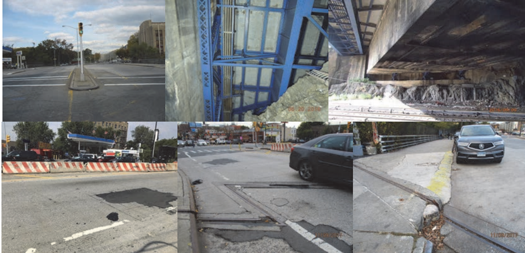
Top of Bridge. June 2016: Roadway Deck Underside of Span 1, Transverse Cracks With Efflorescence and Hollow Sections. (Credit: NYSDOT) September 2016: Southeast Portion of the South Abutment - Underside Framing. September 2017: Jersey Barriers on Beginning Approach. November 2017: Beginning Abutment Joint Northbound Roadway (Right Side) - Depressed Sealant, Missing Armor and Concrete Header. Left Curb Adjacent to Beginning Joint - Missing Steel Face. (November Credit: NYSDOT)
