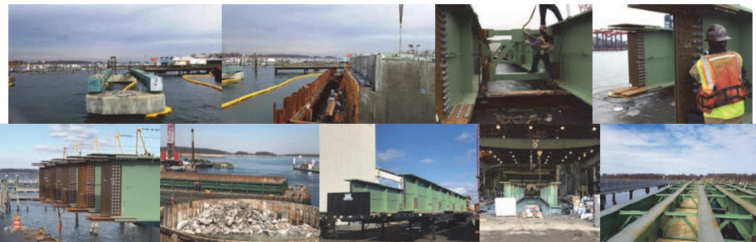
January 2017: Most of the Superstructure of the Old Bridge Removed. New Bridge Abutment Seat That Will Support the New Bridge Deck. Two Girders are Attached With a Diaphragm. A Worker Installs Bolts at the Splice Location Prior to Shipment to the Site. The Bridge Steel Beams Were Installed at the Footprint of the Original Structure. The American Steel was Fabricated in Southfield, New Jersey and Sent to Elizabeth, New Jersey, Where it was Loaded on Barges and Sent to City Island. Upon Arrival, Construction Workers Offloaded the Steel and set it in its Final Place. February 2017. Steel Fabrication. March 2017.
