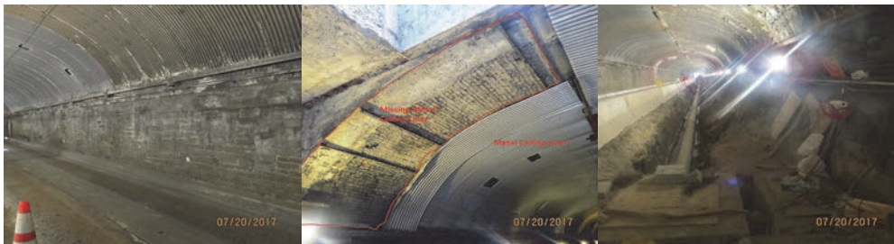
July 2017: West Tunnel Liner, Looking West - Efflorescence and Water Leakage and Missing Mortar Between the Masonry Stones. North Side End of Brick Arch, Looking Southeast - Missing Section of Metal Ceiling Liner and Mortar Between Bricks. East Side of Tunnel, Looking Northeast - Installation of New Drainage Pipe.
