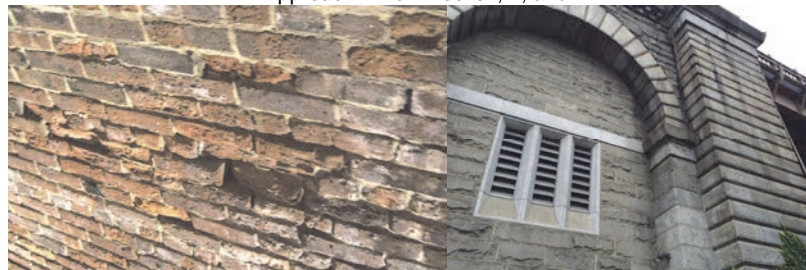
Brooklyn Approach Arch Block I: Deteriorated Brick on the East Face of the Barrel Wall. South Elevation - Staining and Loss of Mortar at the Joints and Arch Stones.
