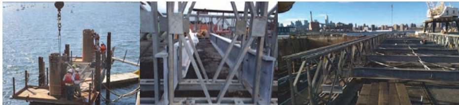
October 2014: The Contractor Airlifted Drilled Shaft Casings Into Position on a Platform Constructed Beside a Construction Barge. The Contractor Assembled the Temporary Bridge Segments at the Brooklyn Navy Yard. The Pieces Were Transported to City Island by Barge.
