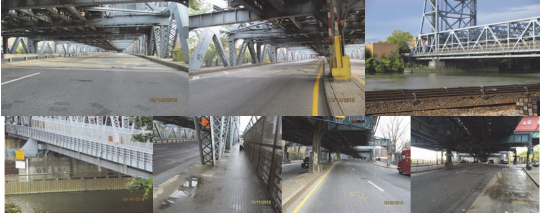
2015: Northbound and Southbound Roadways. South and North Piers. November 2015: Span 2 Right Sidewalk, Beginning and End Approaches, (Credit: NYSDOT)
