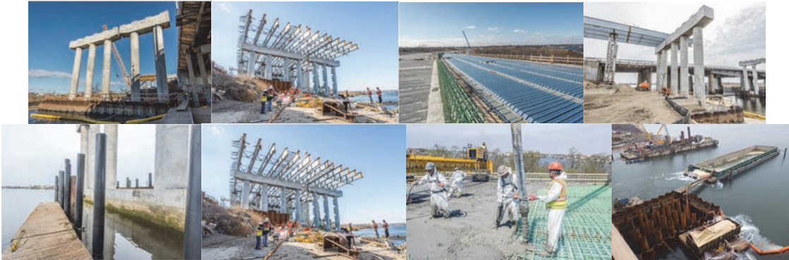
Mill Basin January 2017: Northwest Quadrant Pier #10 - New Columns and Cap Beams in Place. Existing Bridge Columns, Cap Beams, and Deck-Carrying Traffic at Right. Southwest Quadrant Pier #6. Southwest Quadrant Eastbound Deck Preparation at Pier #3 – Epoxy-Coated Rebars for Future Median. Completed Northbound Deck at Left. Stay-in-Place Galvanized Steel Forms at Right. February 2017: Structural Steel Set on Pier #10. The Existing Mill Basin Bridge is in the Background. New Pier #9 at Far Right. Fiberglass Reinforced Plastic Piles for Future Fender System at Pier #9. March 2017: Pier # 6 at the Southwest Quadrant. April 2017: Pumping and Finishing Deck Concrete at Pier #2, Unit 1, Westbound. Dewatering Pier#2 Cofferdam Into Barges to Settle and Filter Water Discharge Into Jamaica Bay.
