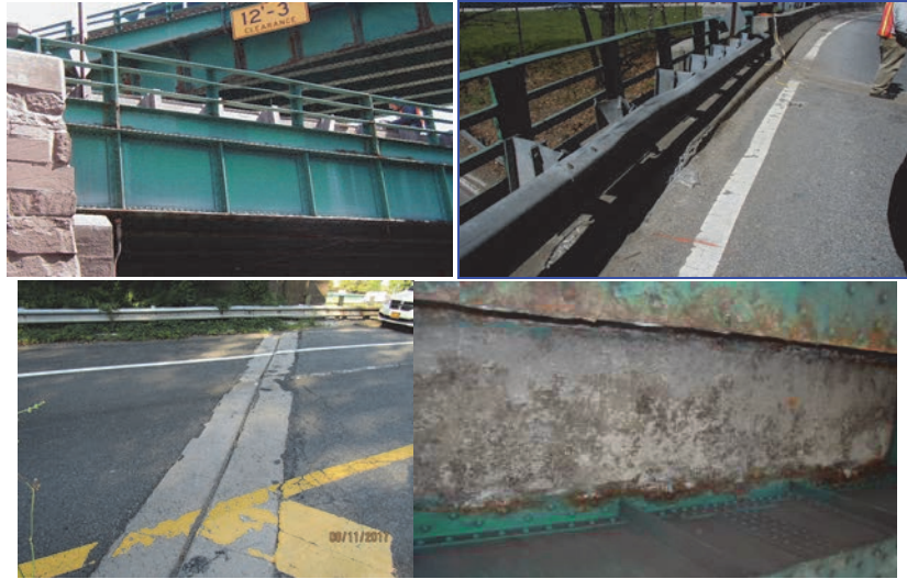
South and North Fascia - Along the Fascias are Built-Up Riveted Steel Girders. The Steel Railing Posts are Welded at the Base to the Top Flange of the Fascia Steel Girders. Deterioration of Joint at Abutment. Underside of Deck with Scaling and Efflorescence.
