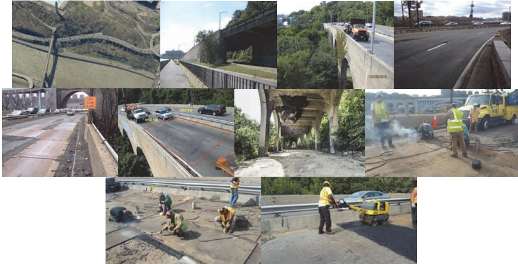
Aerial View. Trans-Manhattan Expressway Connector Ramp in 2014: Elevation Right Spans 1 – 25, 33 – 40. (Credit: NYSDOT) March 2015 Field Inspection. September 2015 - Span 42, Northbound Roadway, Looking Back. (Credit: NYSDOT) November 2015: Netting at Deck Underside. Repairing the Punch Through Holes on Top of the Deck.
