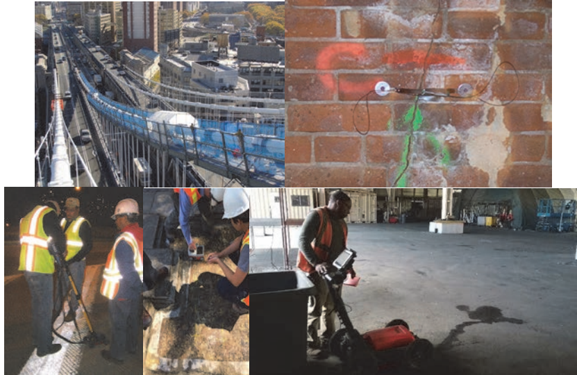
Experimental Corrosion Sensors Installed for a Test on Cable D of the Manhattan Bridge in 2011 (Left Corner). A Fiber Optic Sensor Monitoring a Crack in the Masonry of the Brooklyn Bridge's Manhattan Approach. A Ground Penetrating Radar Inspection of the Belt Parkway Bridge over Ocean Parkway. (Credit: Bojidar Yanev) 2016: Ground Penetrating Radar Utilized to Locate Rebars in the Brooklyn Heights Promenade Pavement. 2017: Ground Penetrating Radar Utilized to Detect Possible Subsurface Voids and Areas of Disturbed Soils That Could Cause Settlement in a Fenced, Paved Maintenance Storage Yard Located Under an Elevated Section of the FDR Drive Near its Intersection With the Avenue C Loop.
