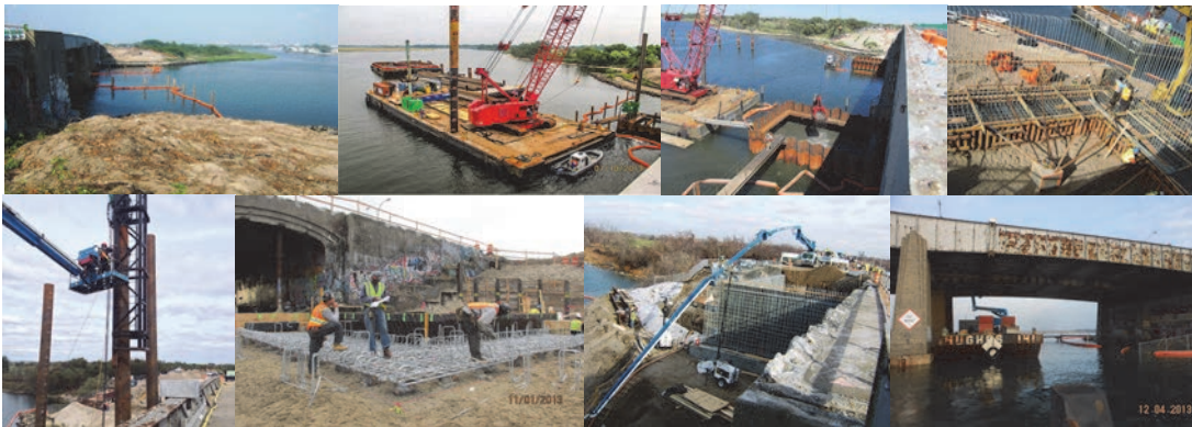
June 2013: North Side of Gerritsen Bridge - Turbidity Curtains Placed on Both Sides of Navigable Channel. July 2013: Work Barges Driving Steel Sheeting for Pier #1 Cofferdam. September 2013: Rebars and Form Work for Footing and Walls at the Northwest Abutment. Stage 1 Piles. October 2013: Inspecting Rebar. November 2013: Tremie Concrete Pour at Pier #2. December 2013: Inspecting Spans 7 and 8 of the Existing Bridge From a Barge. (Inspection Credit: NYSDOT)
