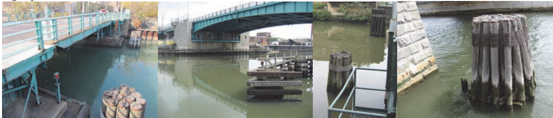
2014: Union Street Bridge Dolphins. Greenpoint Avenue Bridge Dolphin & Fender System. (Greenpoint Credit: Peter Basich) Hunters Point Avenue Bridge Dolphins. (Credit: Michele N. Vulcan) 145 th Street Bridge Dolphin. (Credit: NYSDOT)
