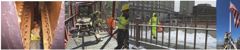
Bridge Repairer Riveter Damian Venezia Squeezing Between the Girders to Access a Floor Beam That Needed to be Reinforced on the Ed Koch Queensboro Bridge – August 2010. (Credit: Hany Soliman) Carpenters John Horgan and Ruben Urena, and Assistant Civil Engineer Fouad Althaibani Repairing the PS-5 Bridge in November 2011. (Credit: Thomas Whitehouse) Cement Mason Victor Porowski Spreading Sodium Acetate on the Walkway of the Brooklyn Bridge in 2013. (Credit: Paul Schwartz). Supervisor Bridge Painter Cesar Pazmino Demonstrating Flag Change Preparations. (Credit: Bonny Tsang)
