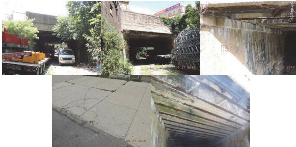
Southern Boulevard Bridge Over CSX. July 2016: Elevation Left and Right. Begin Abutment Stem Exhibits Vertical and Horizontal Cracks With Efflorescence, and Isolated Areas of Hollow-Sounding Concrete. Left Sidewalk at End Abutment. (Credit: NYSDOT) September 2016: Right Side Under Deck of span #1 – Mold is Present and the Bottom Flanges are Corroded.
