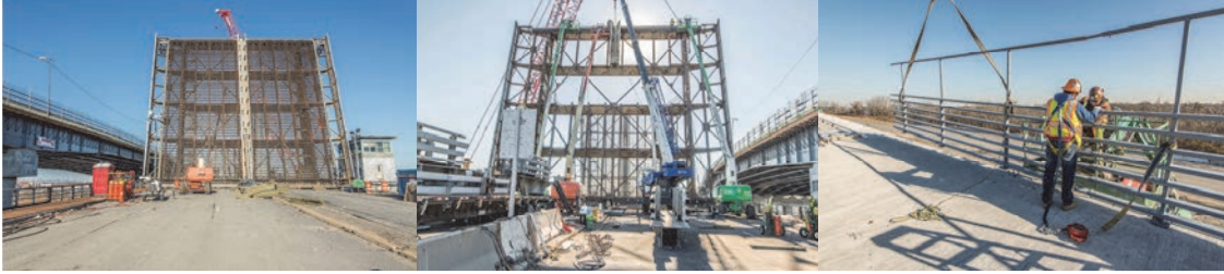
December 2017: South Leaf of the Mill Basin Bridge During Demolition. Sidewalk and Median Removed. The New Bridge is at Left Carrying Eastbound and Westbound Belt Parkway Traffic. North Leaf of the Mill Basin Bridge During Demolition. Steel Bridge Deck, Median, and Walkways are Removed. New Mill Basin Bridge is at the Right Side. Erecting the 7-rail Bridge Rail and Fence at the East Side of the Bridge for the Bicycle/Pedestrian Walkway.
