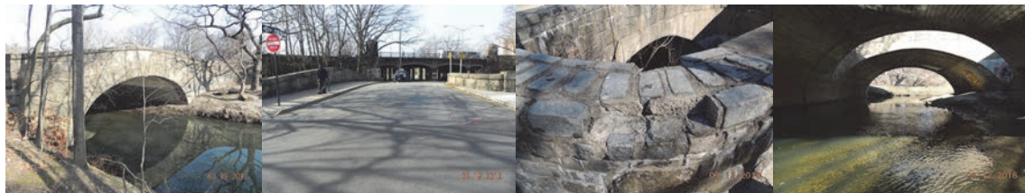
Bronx Boulevard Northbound Bridge Over Bronx River. March 2012: Elevation Right. End Approach. March 2016: Span 1, Left Stone Parapet - Spall Near Beginning Abutment. Span 1, Upstream Channel Looking Left - The Upstream Enters the Underside of the Bridge at a 45 Degree Angle Causing Erosion Along the Left Embankment. (Credit: NYSDOT)
