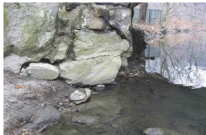
Scour on Pier 2 End Face of Mosholu Parkway Bridge Over Bronx River in 2008. (Credit: NYSDOT)
