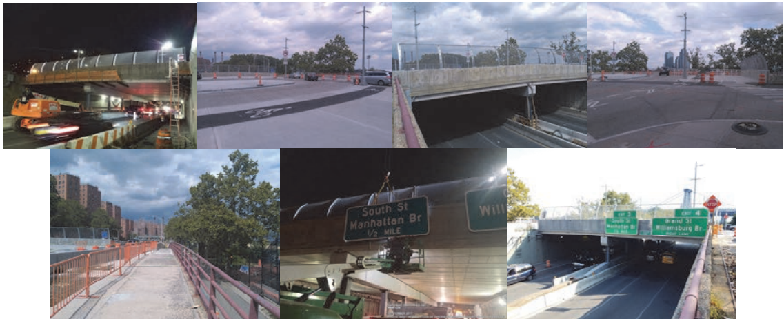
August 2017: Night Work. Overpass Open. September 2017: Installation of Overhead Roadway Signs on the North Parapet.
