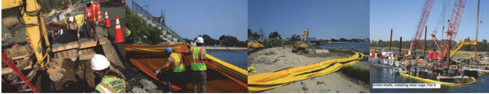
August 2014: Excavating on the West Side of the Bridge in the Presence of an Archeologist. Approximately 300 Linear Feet of a Turbidity Curtain was Installed on the Southwest Side of the Bridge to Protect the Shore During Construction. A Turbidity Curtain is a Floating Barrier Designed to Contain and Control the Dispersion of Sediment. October 2014: Drilled Shafts – Installing Rebar Cage at Pier 6.
