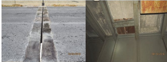
2016: Pier 102, Deck Joint at Southbound Roadway – Missing Joint Sealer Material. Span 143, Underside of Deck – Deep Spall. (Credit: NYSDOT)
