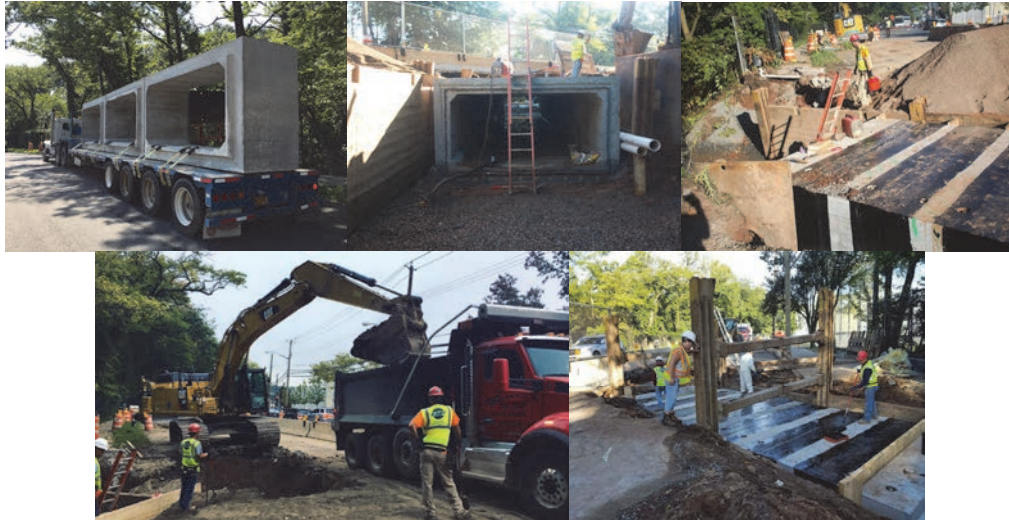
Midland Avenue Culvert in September 2017 – Precast Sections. Looking East - Precast Box Culvert Section Installation Complete. Looking North – Completed Installation of Waterproofing Membrane on the Outside of all Joints. Excavating. Assistant Civil Engineer Tatyana Krushelnitskaya (on Left) Inspecting the Waterproofing of the Culvert Box.
