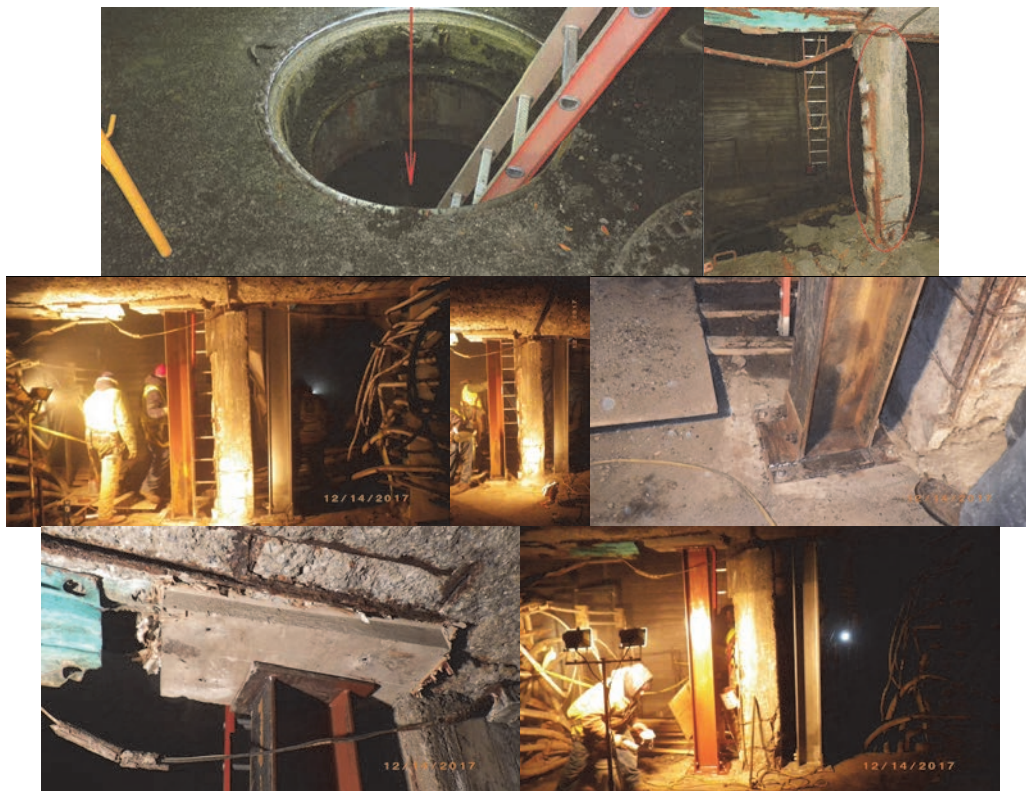
Entrance to the Confined Space. Span 34, Spalled Support Column with Exposed Main Rebars and Broken Stirrups. (Condition Credit: NYSDOT) Repairing the Flagged Conditions.
