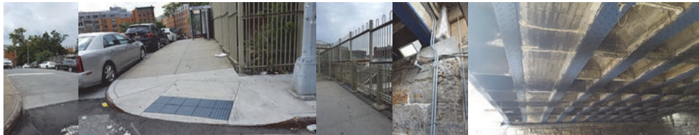
East 162 nd Street Bridge After Construction – New Concrete Overlay. New Southwest Pedestrian Crossing. Repaired Pedestals. Painted Fence and Railing. Sealed Underdeck Cracks.
