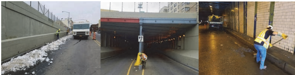
March 2017: Bridge Painters Elisangela Oliveira and Elcio Zaharko Removing Snow From Job Site. Painting the Bruckner Expressway - Bridge Painter Richard Mocciano in September, and Bridge Painter Elisangela Oliveira in October.
