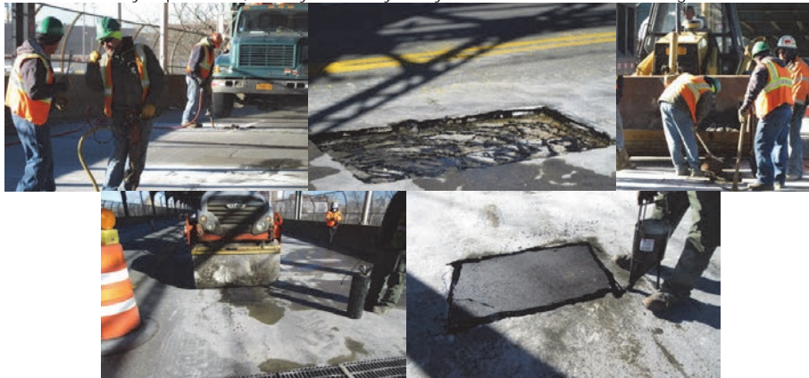
Repairing Potholes on the Roosevelt Avenue Bridge Deck Between Janet Place and 126th Street in January 2016. Each Perimeter is Sawcut. Filling in the Pothole With Asphalt. Paver Rolls Over the Pothole to Compact the Fill Material and Level the Surface. Finished Repair.
