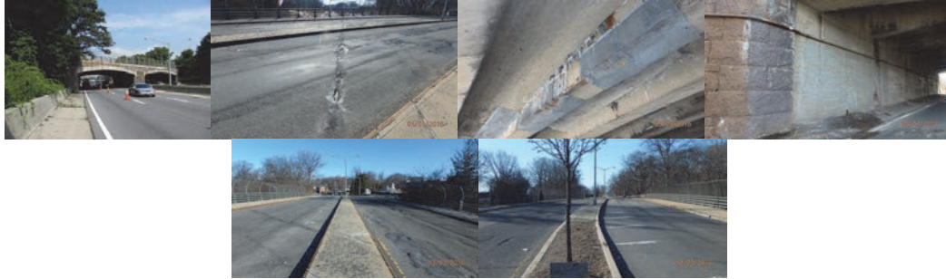
Douglaston Parkway Bridge Northbound Over Cross Island Parkway. March 2016: Top of Bridge, Asphalt Wearing Surface Above Beginning Abutment - Spalls and Uneven Wearing Surface. Span 1 - Deteriorated Concrete Covered With Wire Mesh. Abutment End. Approach Begin and End. (Credit: NYSDOT)
