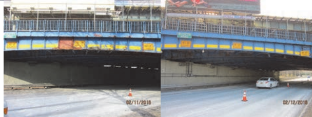
2016: Span 1 Right Sidewalk Near Beginning Abutment – Steel Plates. Girder Reinforced With New Steel Plate and Angles. Strongback Girder at Right Side of Span 1. Right and Left Fascia. (Credit: NYSDOT)
