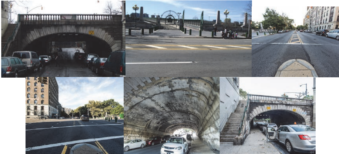
Riverside Drive Bridge over West 138 th Street Before Construction. North and South View, Underdeck, and Stairway.
