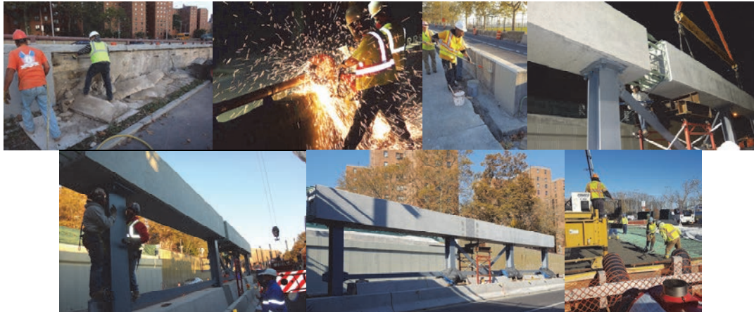
October 2016. November 2016: Stage 2 - Final Bolting and Alignment of Precast Pier Cap Segment. December 2016: Placing and Finishing Concrete for Deck Slab.
