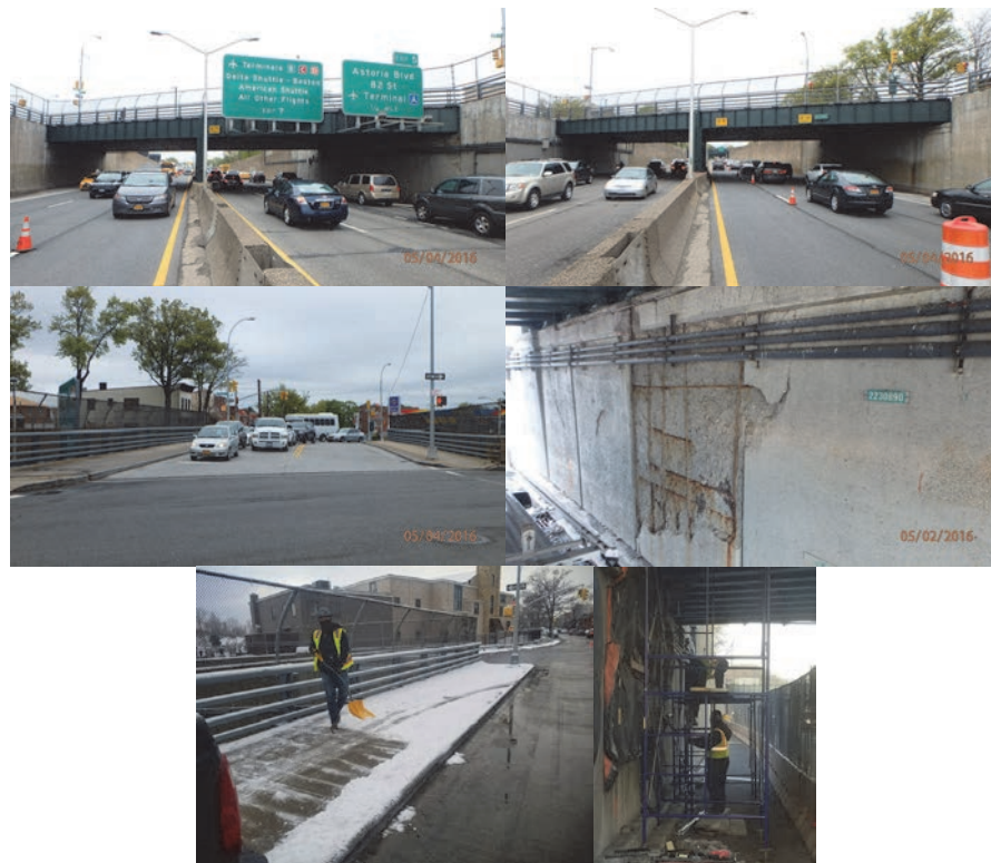
49 th Street Bridge Over Grand Central Parkway. May 2016: Elevation Left and Right. Beginning Approach. Begin Abutment at Bays 9 to 14 - Spalls With Exposed Corroded and Debonded Rebars and Hollow-Sounding Concrete Areas. (Credit: NYSDOT) December 2017: Snow Removal. Erecting Scaffolding at the Abutment.
