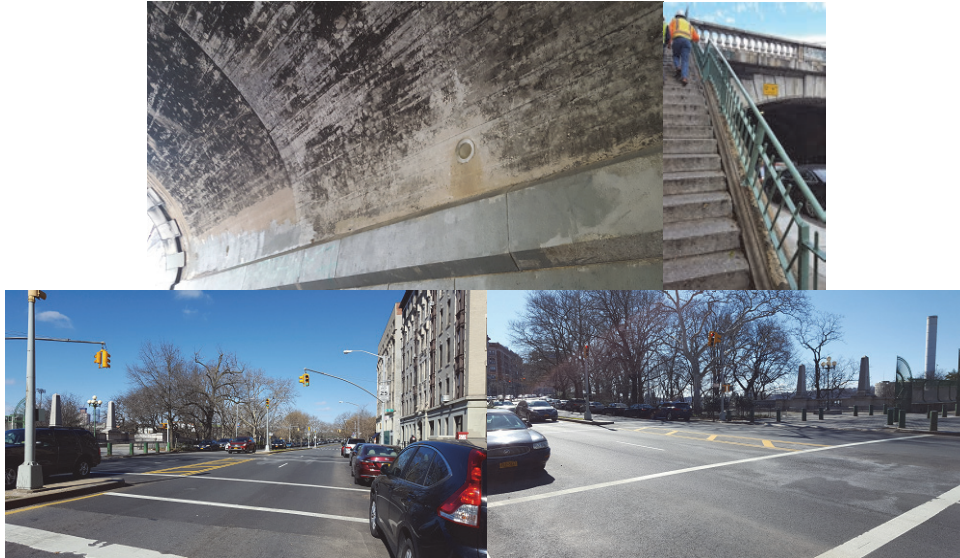
Riverside Drive Bridge over West 138 th Street After Construction – Weep Holes Installed, Railing Painted. New Asphalt Overlay – North and South Views.
