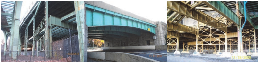
West 72 nd Street Viaduct Left Elevation Spans #1 -5, and Span #107. Piers #3 – 10. (Credit: NYSDOT)
