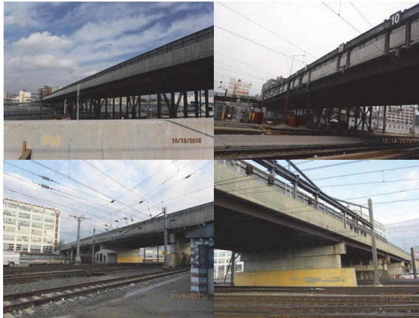
Honeywell Street Bridge in 2015: Left Elevation Spans 6-16. 39 th Street (North) Bridge in 2017: Left Elevation Spans 10-14. Right Elevation Spans 10-12. (Credit: NYSDOT)
