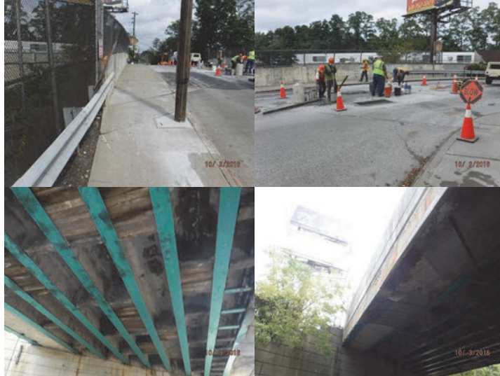
Arthur Kill Road Bridge Over SIRT South Shore. October 2016: Left Sidewalk. Repairing the Wearing Surface at the Beginning Right Side Near the Beginning Abutment. The Wearing Surface has Widespread Cracks and Uneven Asphalt Concrete Patches. Span 1 Underdeck General View of Timber and Wire Mesh Shielding. Stable Hollow-Sounding Areas and Shallow Spalls With Scaling and Efflorescence. (Credit: NYSDOT)
