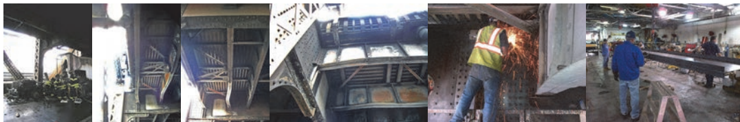
August 2013 - Red Flags on the Ed Koch Queensboro Bridge. A truck caught fire on the bridge and damaged three stringers that support the eastbound upper roadway. Replacement of the two damaged stringers and the repair of a third were completed in October 2013. All work was performed by in-house forces. August 2013: Firefighters Examining the Damage. Repairing the Bridge Included Custom Designing the Steel Beams, as Well as Fabrication and Installation. Division Ironworkers Fabricated Two 26-Foot-Long, 1.5-Ton Beams in Their Brooklyn Shop.
