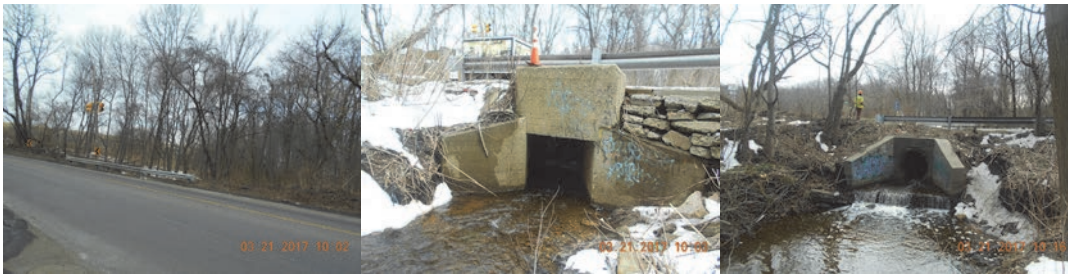
Arthur Kill Road Culvert over Muldoon Avenue in March 2017 - Looking Northwest at the North Side. Looking North at the South Headwall and Wingwall, and Looking South at the North Headwall and Wingwall.
