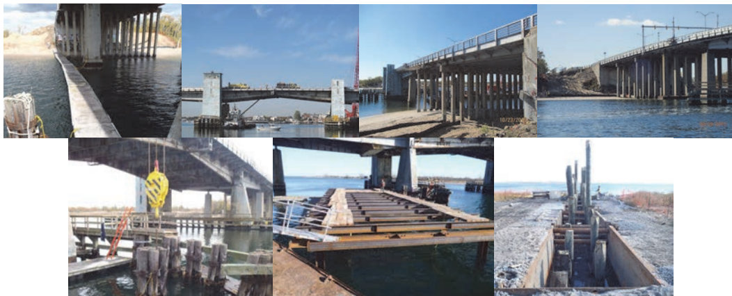
October 2015: Temporary Walkway on North Side of Bridge for Access to Pier #9. Elevation Left Span Elevation Right Span 8, 9-14, 1-7. (Inspection Credit: NYSDOT) November 2015: Extracting Wood Piles From the Existing Bridge Fender System at New Pier #9 Site. Pier #9 Steel Framing for the Cofferdam on the West Side of the Existing Bridge. December 2015: Outfall #2. Pressure Treated Wood Piles – Facing East.
