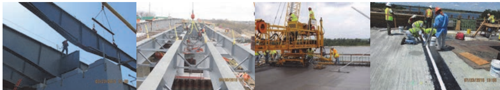
Gerritsen March 2015: Lowering a Girder onto the North Side of Pier #1 - Facing Southwest. April 2015: Four Girders With Diagonal Braces Set Between the East Abutment and Pier #2. June 2015: Placing and Finishing Deck Concrete. July 2015: Placing Armorless Joint in the Deck of the Westbound Bridge.
