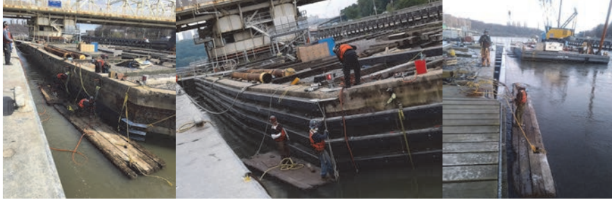
Installation of New Lumber on the Existing Fender. Building an Extension at the Northeast Side of the North Fender with New Lumber.
