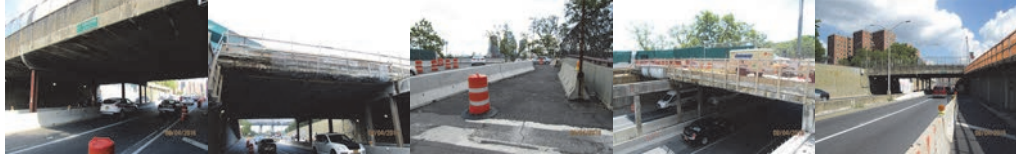
The Three Structures of the FDR Drive at Houston Street Overpass. 2016: Main Bridge – Span 2, Underside of Deck Slab. Partly Removed Deck Slab. Temporary Pedestrian Walkway. Left and Right Elevations in August.
