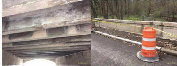
April 2017: Superstructure Framing – Repaired Concrete-Encased Steel Stringers and Concrete Underdeck. Begin Approach, Left Curb - New Segment of Concrete Curb. (Credit: NYSDOT)
