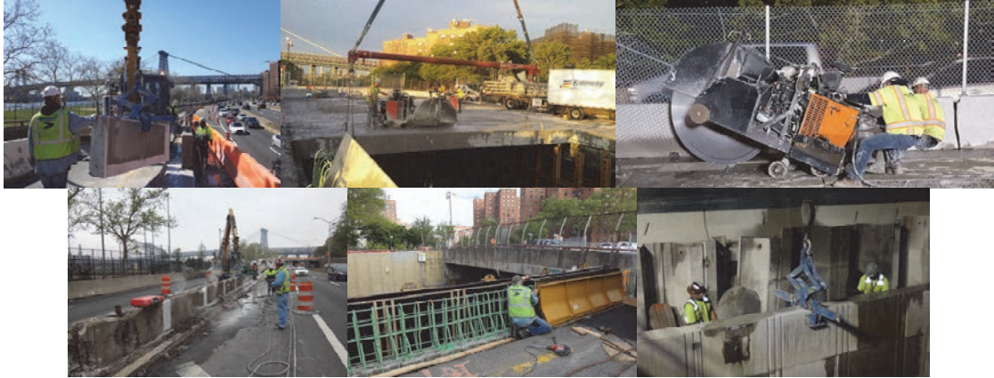
April 2016: Demolition of West Barrier Wall at Exit Ramp. May 2016: Saw Cutting the Existing Deck. Saw Cutting and Demolition of West Barrier Wall at Entrance Ramp. Erecting Forms for West Barrier Wall at Exit Ramp. July 2016: Saw Cutting and Demolition at West Abutment Wall.
