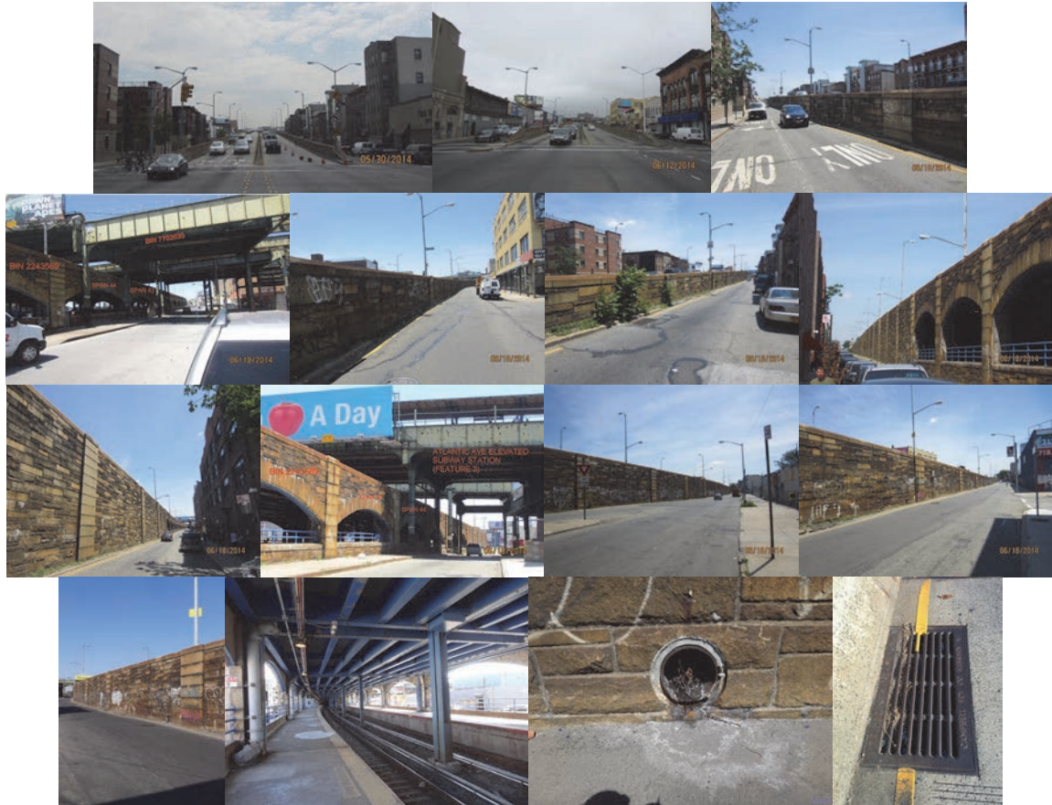
Beginning and End Approaches in 2014. Elevation Left – Spans 1 – 20, 38 – 45, and 50 - 75. Elevation Right Spans 1-20, 5 – 34, 28 – 43, 43 - 52, and 48 - 58. (Credit: NYSDOT) Stone Curtain Wall. Typical Scupper, Downspout and Outlet to Street.
