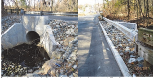
November 2017 – Half of the Culvert is Rehabilitated – Beginning and Ending Approach Right Side Embankments are Repaired. New Guide Railing, Bridge Railing, Curb and New Asphalt Pavement.
