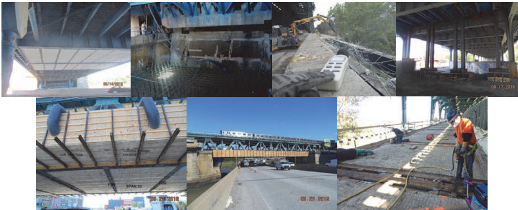
June 2016: Contractor Installs Shield Under the Bascule Span to Prevent any Debris From Falling onto the Van Wyck Expressway or Into the Flushing Creek During the Demolition Process. The Contractor Poured Lightweight Concrete on the Bridge's Counterweight Pits. These Pits, Located on the East and West Sides of the Flushing River, Were Necessary When the Bridge was a Drawbridge. Now That the Bridge is Locked in Place, the Agency Decided to Fill Them with Lightweight Concrete. This Will Prevent Them From Accumulating Water, Reducing a Potential Health Hazard. July 2016: Contractor Using a Robot to Break Through the Existing Sidewalk on the North Side of the Bridge. Using This Technology Reduces the Risk of Injury to Personnel During Demolition and Gives the Operator a Better View of the Actual Demolition. August 2016: Span 6 - Temporary Steel Shoring in Front of Pier 6. Span 20 Left Side - Encased Underside of the Span. Span 20 Elevation Right. (Spans 6 and 20 Credit: NYSDOT) October 2016: West Viaduct – Stage 1 Removing the Original Bridge Deck.
