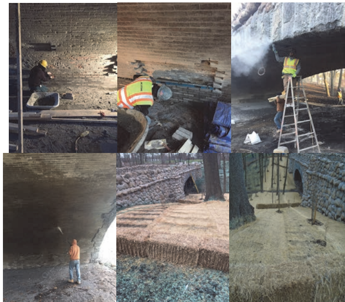
April 2017: Installing the New Underside Bricks - Matching Bricks in Color and Dimensions. Power Washing Under the Arch. Erosion Control Material Placed Over the Bridge Slope.
