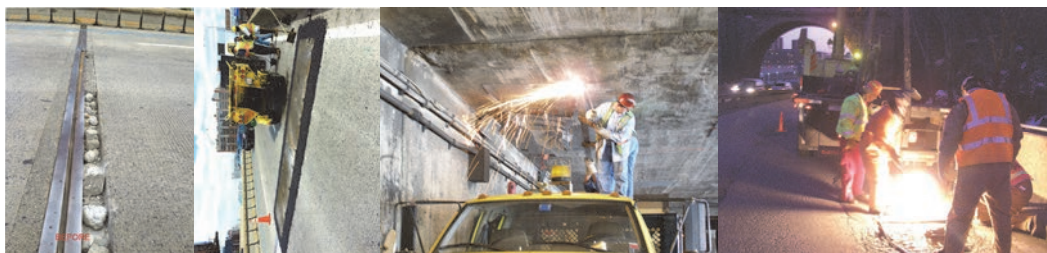
August 2014 PIA Safety Flag: Broken Joint Concrete Header And Steel Armor on the Long Island Expressway over Dutch Kills Creek. The Condition Was Made Safe By Installing Two Steel Plates. PIA Flag (Truck Wedged Under the FDR Drive at Span 41): Removing the Debris. (Credit: Victor Sandoval) PIA Flag Repair (Through Hole) on Harlem River Drive Ramp. (Credit: Bojdar Yanev)
