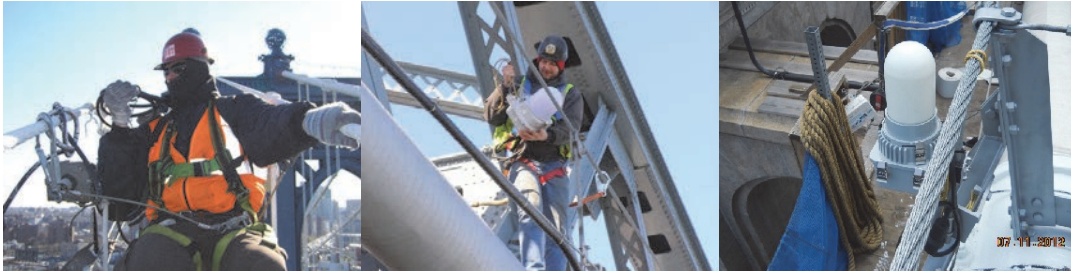
Repairing a Manhattan Bridge Necklace Light. Bridge Repairer and Riveter Neil Dalton Installing a New Light on the Williamsburg Bridge in 2012. (Credit: Hany Soliman) Manhattan Bridge Side Necklace Light. (Credit: NYSDOT)
