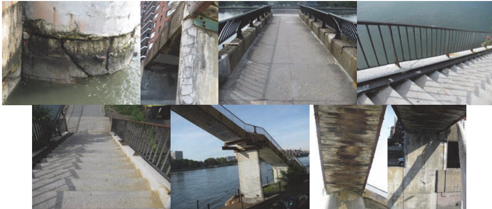
Bridge Conditions in June 2014. Pier 1 Over the East River – Close-up of 2 Wide Cracks. Begin Abutment Stem Right Side - Failing Patch and Map Cracking. Span 1 Deck Wearing Surface. Span 2 Railing. Span 3 Concrete Steps. Pier 2, Under Span 2, Looking Southwest – Spalled Concrete Area With Exposed Rebar at Bottom of Pier. Underdeck of Span 1. Begin Abutment Stem.
