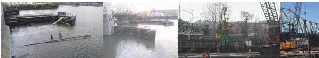
May 2015 – University Heights Collapsed Fender System. Collapsed Fender System in East Channel. December 2015: Loosening the Existing Wooden Pile to Facilitate its Easy Removal From the River (Mud) Bed. The Vibrating Hammer is Attached to the Crane Initially to Vibrate it and Ultimately Loosen the Existing Piles. . April 2016: Pile Driving Operation.
