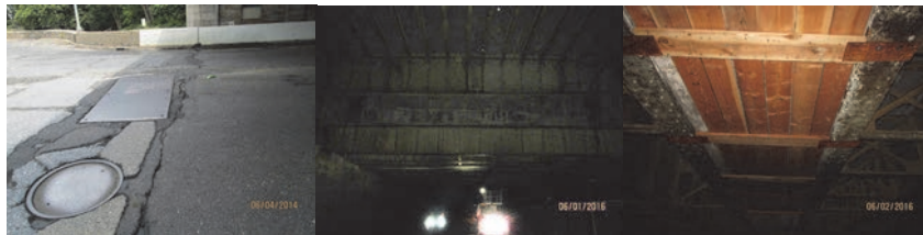
West 79 th Street Bridge Over Amtrak in 2014 – Beginning Abutment Joint – Top of Deck. June 2016: Left Elevation. Underside of Deck, Bay 7 – Timber Shielding. (Credit: NYSDOT)
