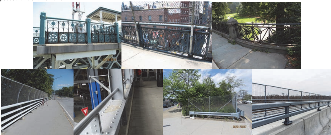
University Heights Bridge Railing. (Credit: NYSDOT) Manhattan Bridge Railing. (Credit: Russell Holcomb) Greywacke Arch Guide Railing in 2017. Northern Boulevard over Cross Island Parkway - Left Sidewalk Railing in 2016. Staten Island Pedestrian Bridge over Parking Lot Exit Roadway - Right Side Railing of Span #2. 14th Avenue Bridge over Cross Island Parkway -End Approach Guide Railing in 2017. New Belt Parkway Bridge over Mill Basin Guide Railing.
