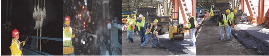
Power Washing the Corrosive Deicing Solvents Within the Range of the Roadway Splash Zone on The Manhattan Bridge in October 2007. Particular Attention is Directed to Cleaning the Gusset Plate. (Credit: Albert Hong) Performing Wear and Tear Resurfacing Work on the Roosevelt Avenue Bridges in April 2010: Assistant City Highway Repairer Victor Magagna, Supervisor Highway Repairer Joseph Palemine, Assistant City Highway Repairer Jonathan Adorno (Obscured), Assistant City Highway Repairer Anthony Montalbano, and Area Supervisor Highway Maintenance Edward Pedersen. Assistant City Highway Repairers Jonathan Adorno and Victor Magagna. (Credit: Joseph Flood)
