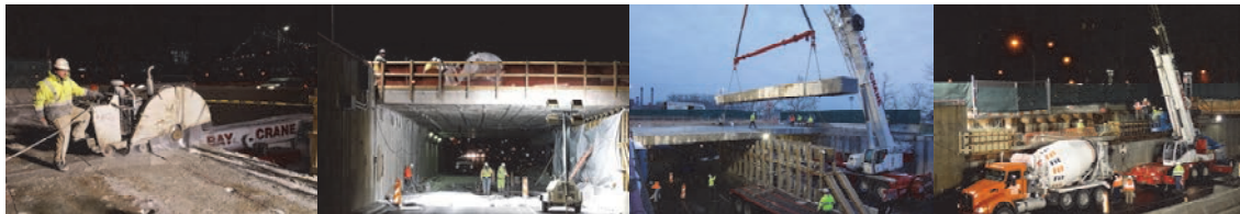
February 2017: Full Depth Saw Cutting of Deck Panels. Stage 3 - Protective Safety Shielding Over Highway. Loading of Deck Slab Panels for Disposal Off-Site. March 2017: Concrete Placement at West Abutment Wall Seat.
