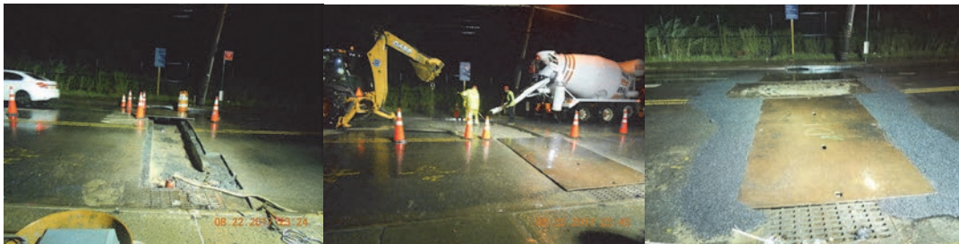
Arthur Kill Road Culvert over Ridgewood Avenue in August 2017 - Cut Back Asphalt Wearing Surface. Placing Concrete Base. Plates Installed Over Trench for the New 20 Inch Diameter Iron Pipe.
