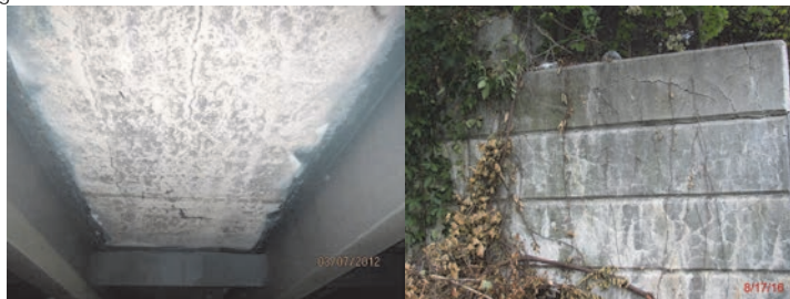
Union Street Bridge over Brooklyn-Queens Expressway in 2012 – Extensive Map Cracking With Efflorescence on the Underside of the Deck. (Credit: NYSDOT) Tompkins Avenue Bridge over B&O Railroad (Abandoned) in 2016 - Map Cracks With Efflorescence Near the End of the Wing Wall.
