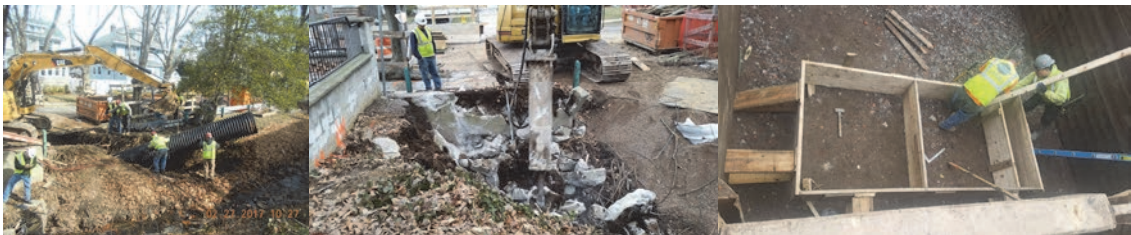
Gregg Place Culvert in February 2017. Looking Northeast - Installation of 30 Inch Pipe for Water Diversion Structure. March 2017 - Looking South - Forming up Footings for the Headwall.
