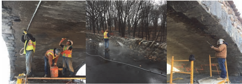
January 2017: Tuck Pointing the Bricks. Power Washing the North Parapet Wall. February 2017: Underdeck Brick Removal - the Extent of the Deteriorated Bricks was Not Known Until Multiple Layers of Existing Paint Were Removed From the Underside Surface of the Bridge Arch.
