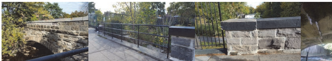
East 180 th Street Bridge After Construction – South Wall, New Railing at South Sidewalk, North Parapet Wall, and Sealed Underdeck Cracks.
