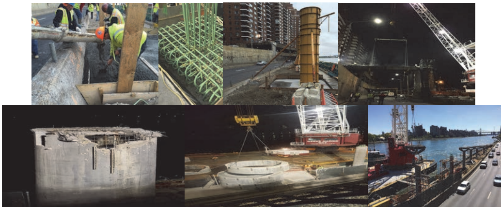
Installing Rebar Cages and Pouring Concrete for Pile Caps. Installing Pier Caps and Removing the Old Bridge. Demolishing the Concrete Tower. Installing the Hub and Arms. (Credit: NYCDDC)
