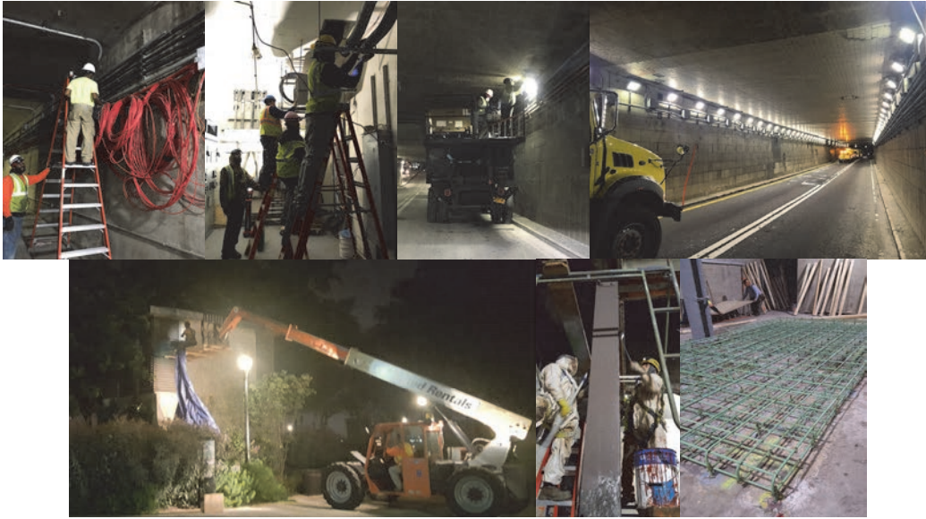
Battery Park Underpass – June and November 2017 – Installation of Cables and Conduits. January and July 2017: Lighting Fixture Repairs. August 2017: Surface Preparation for Turning Vane Painting. Intumescent Painting Application. October 2017 – Placement of Reinforcement for the New Fans' Bases. (Credit: Darlyn Alvarez)
