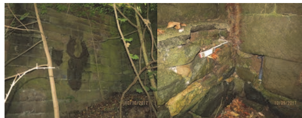
Hill Drive Bridge in 2017: Span 1, Left Exterior Enclosed Wall. End Abutment, Stones on Left Wingwall – Void Due to Missing Stones. . (Credit: NYSDOT)
