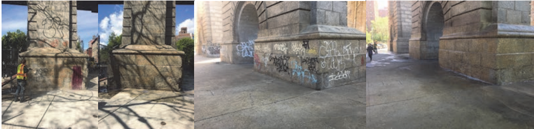
May 2017: Bridge Painter Matthew Somers Removing Graffiti on the Manhattan Bridge. Before and After. (Credit: Herbert Rodriguez)
