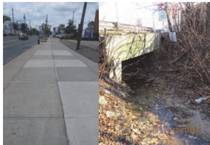
Forest Avenue Culvert over Crystal Avenue in July (Left Sidewalk Looking West) and December 2017.
