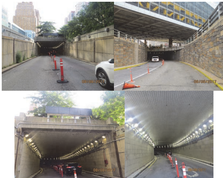
August 2017: West Street Underpass Elevation North and South. North Concrete Portal. Variable Message Board Will Be Replaced.
