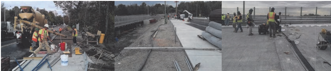
October 2017: West Approach Roadway – Placing Concrete at the North Approach. Installing Fencing Along the South Sidewalk. Bridge Deck – Completing the Installation of the Modular Joints.
