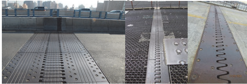
Manhattan Bridge Finger Dam. (Credit: Jagtar Khinda) Unionport Bridge Finger Dam at Span 9 in 2016. Riker's Island Finger Dam.
