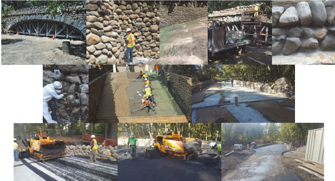
August 2016: Temporary Support Structure Under the Arch. Chipping Out Existing Mortar. Top of Arch - Layout of Epoxy-Coated Mesh Reinforcement and Dowels. South Fascia – Cleaning the Existing Stone. South Fascia Parapet - Finished area – Cleaning, Chipping, and Repointing. September 2016: Wet Burlap Placed Over Previously Finished Zones. September 2016: Center of the Bridge - After Backfilling, the Concrete Base for the Roadway was Placed. Following the Curing of the Concrete Base, Asphalt was Placed.
