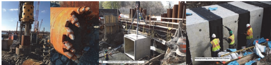
January 2015: Drilling Rig Construction Vehicle Used to Install Land-Based Drilled Shaft Casing for the Temporary Bridge. The Bucket Drills Carve Out the Casings With Teeth Capable of Tearing Through Rock. April 2015: Turtle Cove Culvert Replacement. Installing Culvert Under the Utilities. May 2015: Waterproofing the Joint.
