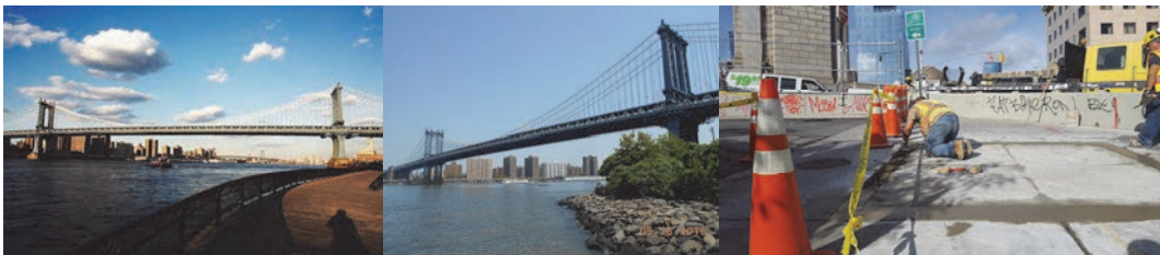
Manhattan Bridge in 2014 and 2016. (Credit: NYSDOT) October 2017: The Bicycle Path was Narrowed but Open While a Division Bridge Repair Crew Repaired the Manhattan Side of the Path.
