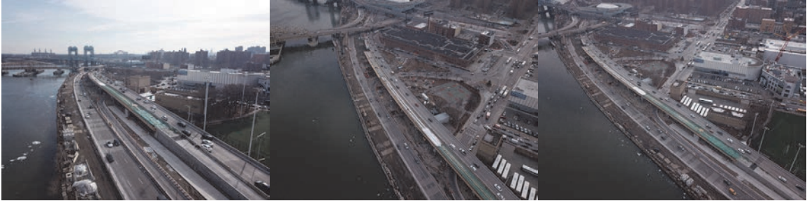
Drone Views: View South - Maintaining all Travel Lanes During Construction. View South From Above Bridge – Willis Avenue Bridge at Upper Left. View of Temporary Roadway for Northbound Traffic.
