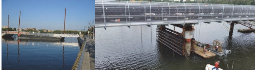
2005: Pontoon Bridge Used During the Emergency Reconstruction of the Ocean Avenue Pedestrian Bridge over Sheepshead Bay. (Credit: Russell Holcomb) 2015: City Island Temporary Bridge.
