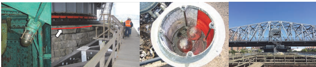
Inspection in Late 2012: Union Street Bridge – Standing Water in East Span Maintenance Light. Madison Avenue Bridge - General View of Fender and Center Pier—the Red Line Depicts the Approximate Water Level. Macombs Dam Bridge – Pier Lighting Fixture with Cover Removed – Silt Deposit on Lamp Tops, and Corrosion on the Fixture Frame. 145 th Street Bridge in August 2015. (Credit: Lity Barreto)
