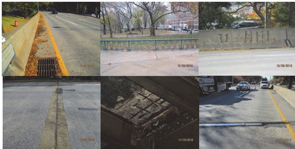
West 94 th Street Viaduct – 2015: Span 34 Left Lane. Span 12 Right Railing and Left Side Concrete Parapet. Span 31 Top of Deck. 2016: Span 4 – Spall With Exposed Rebar. Pier # 3, Deck Joint, Northbound Henry Hudson Parkway, Left Lane – Joint Missing Metal Plate. (Credit: NYSDOT)
