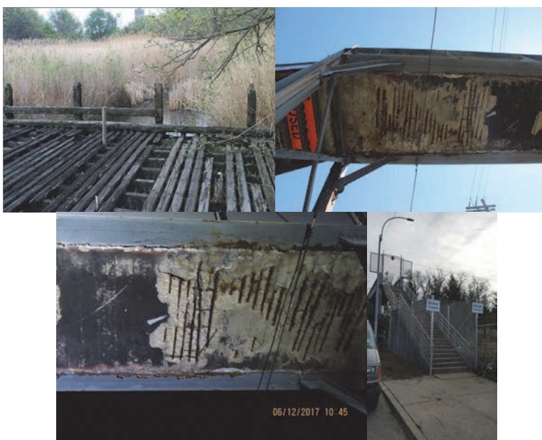
Flushing Meadow Park Pedestrian Bridge – (Date Unknown). 216 th Street Pedestrian Bridge in April 2016: Delaminated Concrete and Detached Exposed Rebar at Span 4 – Deck Underside. June 2017 – Close-up of Span 4. Bridge Closed Sign.
