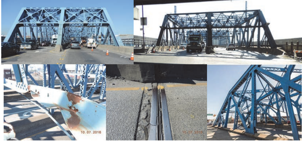
Leggett Avenue Bridge over Amtrak Before Construction. October 2016: Begin and End Approaches. Span 1, Bottom Sway Strut Bracing Exhibits Severe Deformation and Several Upward Bent Sections due to Vehicular Impact. End Abutment Transverse Deck Joint Steel Armor is Cracked. Deck Joint Header Exhibits Shallow Spalls. (Credit: NYSDOT) Southeast View.
