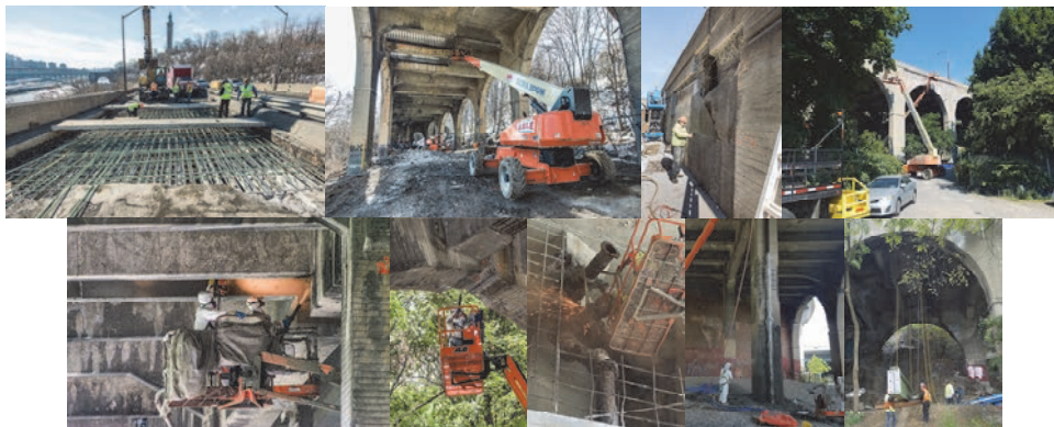
January 2016: Spans 42 and 43 Northbound Rebar Installation. Underside View. March 2016: Pier 3 Concrete Repairs. July 2016. August 2016: Shotcrete Application at Span 36. Chipping at Span 45. September 2016.
