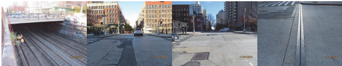
East 97 th Street Bridge over Metro North. 2016: Beginning and Ending Approaches. Beginning Abutment Joint - Deteriorated Sealer Material. (Credit: NYSDOT)
