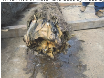
During the Demolition of the North End of the Existing University Heights Bridge Fender, Marine Borers were Discovered in the Southern Yellow Pine Piles. The End of a Pile Segment Removed From the Fender - Based on the Size of the Holes, Teredo Navalis is the Likely Species.
