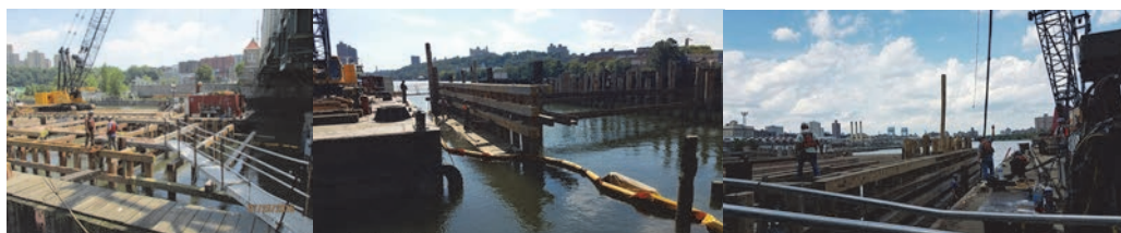
University Heights Bridge in July 2016: Pier 3, Left Side, Repaired Wooden Catwalk. (July Credit: NYSDOT) September 2016: Installing and Securing the Whaler Timbers at the South and East Faces of the Fender.
