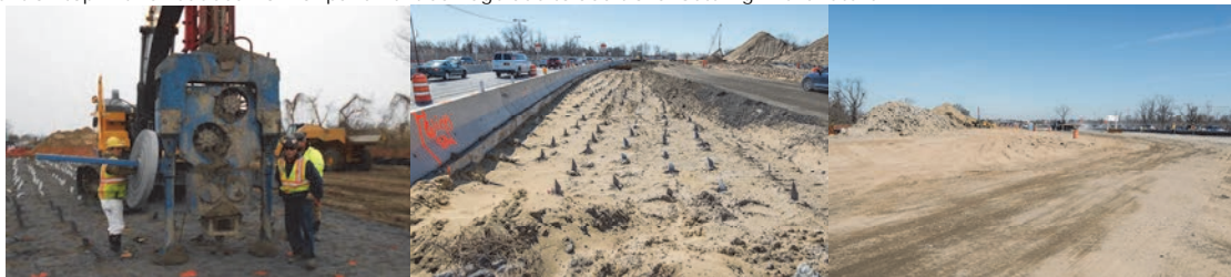
Northwest Quadrant Wick Drains for the New Mill Basin Bridge. Drains Backfilled.
