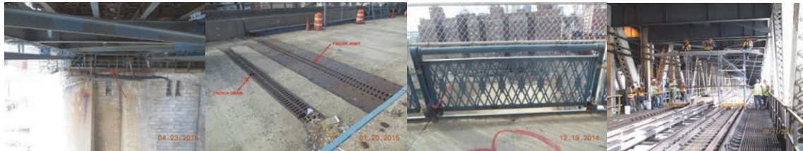
Manhattan Anchorage Maintenance Platform. Looking Northeast at a Trench Drain and Finger Joint on the Parking Deck. First South Rail at South Walkway. 2016: Inspecting the Bridge Using a Rolling Platform. (2016 Credit: NYSDOT)
