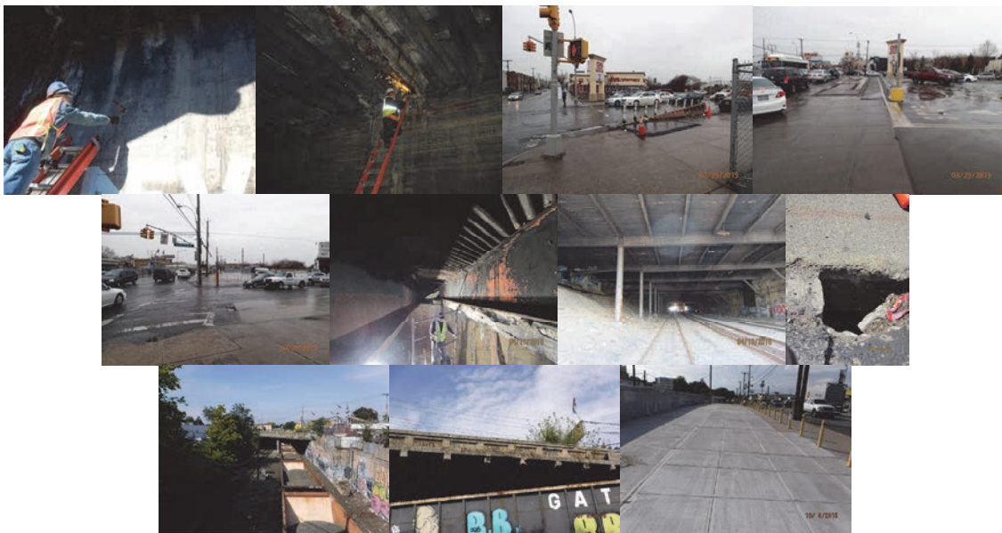
2010 Inspection - Hands-On Inspection of a Pier. Obtaining a Steel Coupon Sample From a Stringer. March 2015: Looking West, South, and East Across Bridge Deck. April 2015. October 2015: Elevation Right. Span 2 Right Parapet - The Outer Face Exhibits Spalls With Exposed Rebars. Spans 1 and 2 New Right Side Sidewalk. (Credit: NYSDOT)
