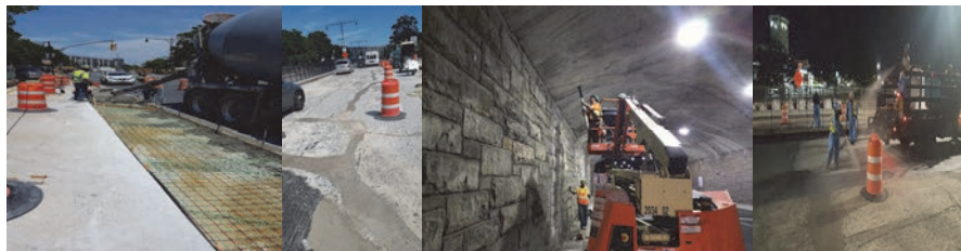
Southern Boulevard Bridge During Construction – Sidewalk Repair, Deck Repair, Weep Hole Installation, and Waterproofing.
