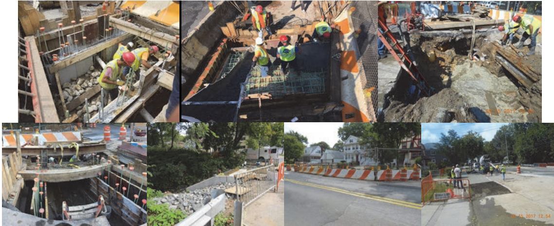
August 2017 - Looking Northwest - Constructing Falsework to Support the Culvert Roof Slab. Pouring Concrete for the Stage 2 Roof Slab. Contractor Excavated and Demolished the Existing Culvert for the Final Stage Along the South Side of Forest Avenue. September 2017 - Concrete Placement at Culvert Walls. Construction of Culvert Opening. Temporary Barrier. Looking West - Contractor Placed Concrete for the Sidewalk, and Seed and Topsoil at Unpaved Areas.
