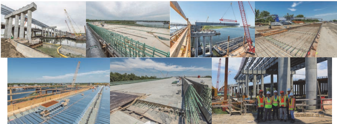
Mill Basin May 2017: New Mill Basin Bridge Columns, Cap Beams and Structural Steel in Place at Pier #10 Over the Navigable Channel. Old Mill Basin Bridge Carrying Belt Parkway Traffic is in the Background. Wet Cure of New Concrete Deck Over Pier #5. Epoxy-Coated Barrier Rebars in the Foreground. June 2017: Erecting Structural Steel in Northwest Quadrant Between Pier #8 and Pier #9. Placing P.C.C. Pavement at the Approach to the Bridge Utilizing a Conveyor. Pavement Forms, Reinforcing Mesh and Joint Dowels are in the Foreground. Stay-in-Place Galvanized Steel Forms, Shear Studs and Scupper in Place for Future Deck Concrete Placement. Westbound Roadway and Barrier. FHWA Site Visit and Project Review: Jason Lin (NYSDOT), Senior Area Engineer Region 11 Richard Beers (FHWA), Area Engineer Region 5 Lorin Willett (FHWA), King Fong (NYSDOT), Administrative Engineer Daniel Hom, and Associate Project Manager Jessica Wang.
