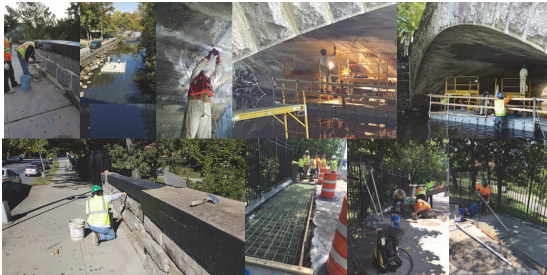
East 180 th Street Bridge During Construction – South Parapet Wall, Working Platform, Crack Repairs, and Tuck Pointing. Sidewalk Repairs.
