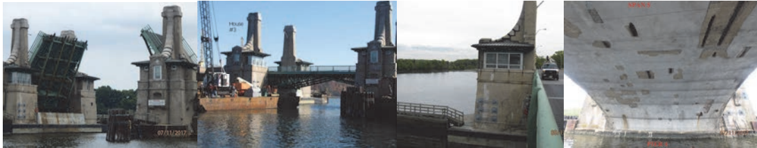
Bridge Open in July 2017. (Credit: NYSDOT) General View of Bridge Operator House #3 in 2011. Bridge Operator House #3 Exterior Wall in 2016, Looking Northwest. July 2017: Underside of Arch Span # 5 - Spalled Concrete With Exposed Rebar is Secured With Netting.
