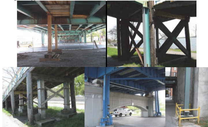
2014: Timber Shoring at Spans 7 and 8 of the Harlem River Drive over Ramp to and From Northbound Harlem River Drive. Steel Shoring of the Damaged Column at Pier 4 of the Crocheron Park Pedestrian Bridge. Timber Shoring at Piers 5 and 6. 2016: Steel Shoring at Span 5 of the East 174 th Street Bridge over the Sheridan Expressway. Eastbound Brooklyn-Queens Expressway over Washington Street - Shoring on the Right Side of the End Abutment.
