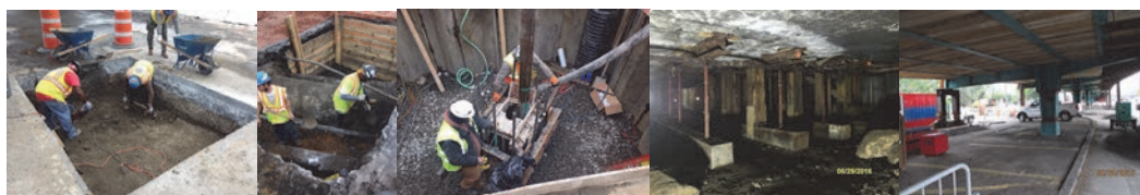
June 2015: Locating and Removing Utilities. (Credit: Artemio Angeles) December 2015: Test Pit Pier 6. January 2016: June 2016: Span 1 Temporary Timber Shoring Under Slab. Span 3 – Timber Planking at Deck Underside. (June 2016 Credit: NYSDOT)
