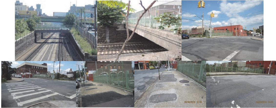
East 175 th Street Bridge View Looking South and North. Top of Deck Looking East and West. Sidewalk and Road Conditions in 2016.
