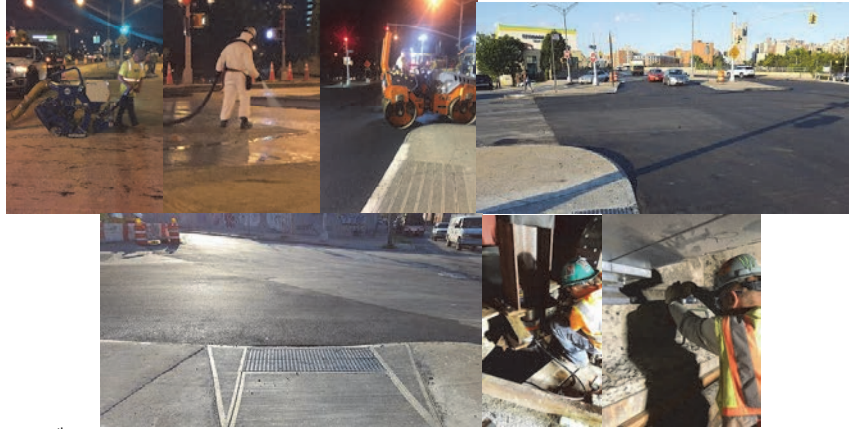
East 165 th Street Bridge Under Construction. Summer 2016. Asphalt Placement. New Pedestrian Ramp. Bridge Jacking. Bearing Replacement.
