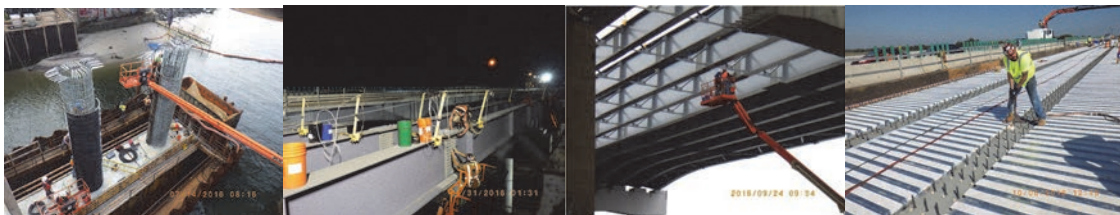
July 2016: Pier #2. Placing Pier Column Forms Around Galvanized Steel Rebar Cages on Top of Plinth. August 2016: Placing High-Strength Bolts Through Girder Splice Plates. September 2016: Torqueing Girder Web Splice Plate Bolts. October 2016: Welder Attaching Shear Studs to the Top Flange of the Eastbound Bridge During Stage 2.
