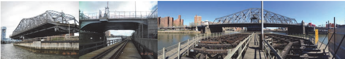
General View of Truss Swinging in 2010 and Right Elevation of Span 15 in 2012. (Credit: NYSDOT) North Elevation View.
