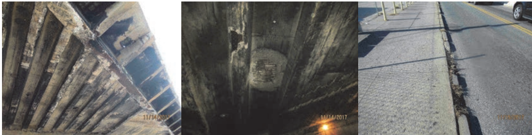
Span 2, Underside of Deck- Spalled Concrete Encasement and Deck. Exposed Rebar. Span 2, Top of Deck - Spalled and Missing Sections of Curb With Vegetation Growth. (Credit: NYSDOT)
