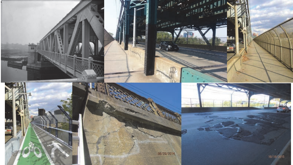
Roosevelt Avenue Bridge – In 1927. (Credit: NYC Records). Looking East. Existing and Proposed Bicycle/Pedestrian Path. 2014: Right Wingwall at the End Abutment. The Top Exhibits an area of Diagonal Cracks With Efflorescence and Spalls. The Deteriorated Concrete Areas are in Safe and Stable Condition. 2015: Spans 26 and 27 – Examples of Uneven Asphalt Patches and Broken Concrete Areas. (Credit: NYSDOT)
