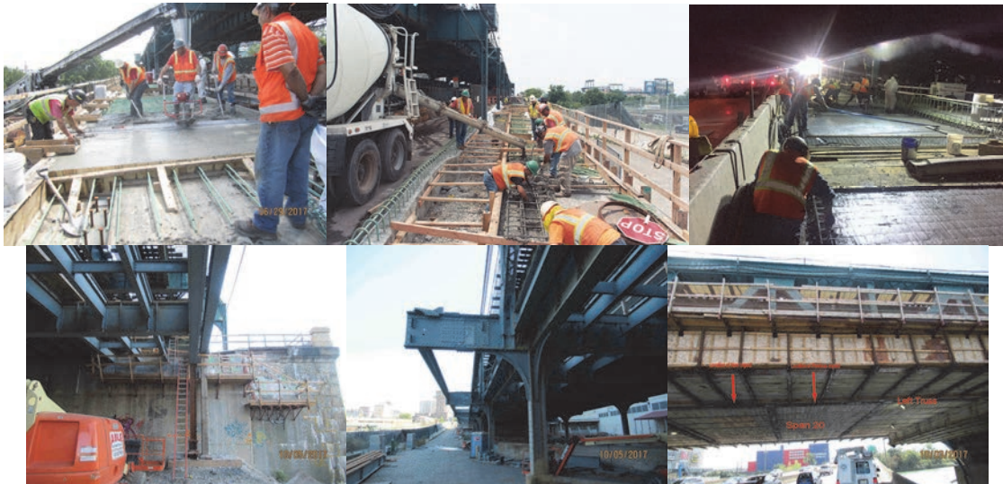
June 2017: West Viaduct – Stage 1 Placing the Sidewalk. August 2017: East Approach – Stage 1 – Placing Sidewalk Concrete. October 2017: West Viaduct – Stage 1 Filling the New Roadway Grid Deck With Concrete. Span 22. Span 20, Left Side, Impact Damage Location. (Spans 20 and 22 Credit: NYSDOT)
