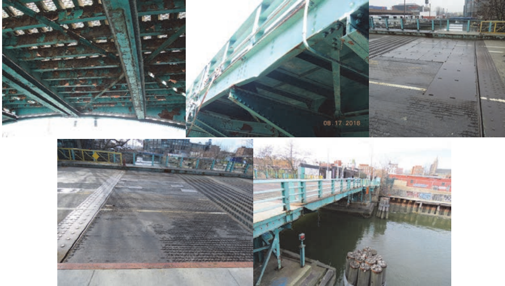
Union Street Bridge - 2016: Severe Corrosion and Peeling Off Paint Under Deck of Span #3. Span 3 - The Left Fascia Stringer Exhibits Impact Damage. (Impact Credit: NYSDOT) April 2017: Steel Plates Covering the Steel Grid Deck. December 2017.
