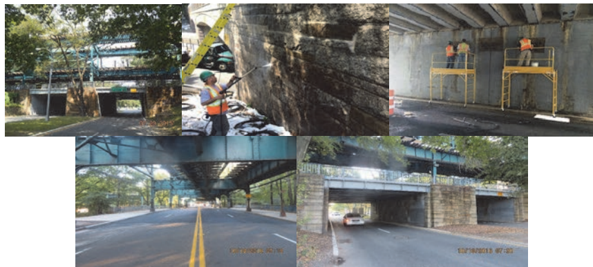
Roosevelt Avenue Bridge in July 2015: Elevation Right. (Credit: NYSDOT) Before, During (Stone Masonry Preparation, Underdeck Concrete Repair), and After Construction.
