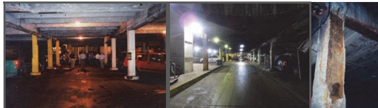
Garage Level – Debris Nets Below Ceiling. Column With Spalled Concrete Encasement.
