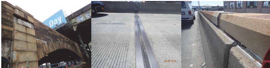
May 2016: Span 43, Right Side Fascia - the Stone Masonry Curtain Wall Exhibits Localized Moderate to Heavy Efflorescence Formation at Several Mortar Joints at the Outside Face and at the Underside of the Arch. Pier 19 Joint, Atlantic Avenue Westbound - Approximately 40% Length of Joint Compression Seal is Slightly Debonded. Spans 33 thru 35, Top of Deck, Right Fascia at Right Bridge Railing - Separation (up to 2") of the Fascia Stones From the Bridge Railing. (Credit: NYSDOT)
