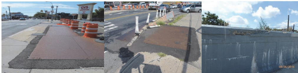
August 2016: Span 2 Left Sidewalk Looking South - Location of the Through Hole. Span 1 Right Sidewalk Looking North. Spalled and Cracked Areas on Top of Span 2 Parapet. (Parapet Credit: NYSDOT)
