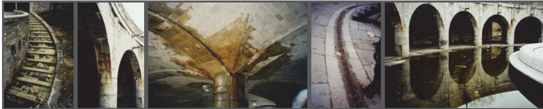
Pedestrian Plaza Level: South Stairway - Deterioration and Missing Stone Steps. Stone Clad Columns - Extensive Efflorescence and Staining. Guastavino Arch - Ponding Water and Efflorescence. Fountain Trench Drain - Deteriorated Grating and Clogged Drain. Extensive Water Ponding.
