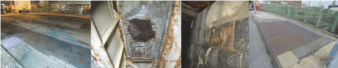
April 2016: Span 1, Wearing Surface at Mid-Span – Uneven Asphalt Patches on Approximately 40% of the Surface Area. Underdeck of Span 1- Through Hole and a Deep Spall With Exposed Rebar Near the End Abutment. There is a Steel Cover Plate Above. (April Credit: NYSDOT) February 2017: Beginning Abutment Masonry Stem Exhibits Missing Mortar Joint. September 2017: The 3 Steel Plates on the Left Sidewalk.
