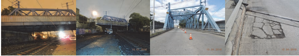
Unionport Road Bridge Over Amtrak – CSX. October 2016: Elevation Left and Right. Beginning Approach. End Approach, Top of Roadway at Right Truss- Exhibits a Spall and Joint Exhibits Torn Sealant. (Credit: NYSDOT)
