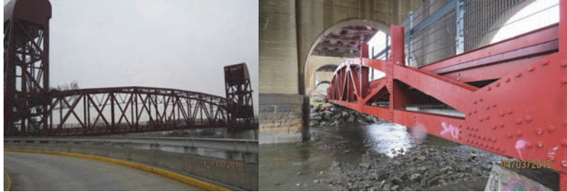
Elevation View of Roosevelt Island Bridge. (Credit: NYSDOT) Right Elevation of Span 3 of the Randall's Island Connector Bridge over the Bronx Kill.
