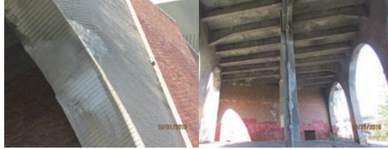
October 2016: Span 51, Underside of Right Arch - Concrete Repairs. Pier 49, at Center Column - Concrete Repairs. (Shielding and Repair Credit: NYSDOT)
