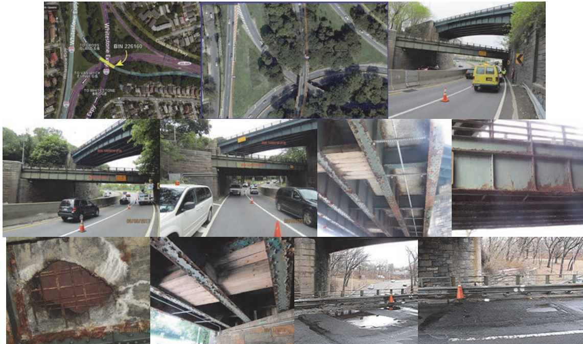
Location Map. (Credit: NYSDOT). Aerial View. Bridge (Lower Structure) in April 2017. Left and Right Elevations in August 2017. (Elevation Credit: NYSDOT) Underside of Span #1 in April 2017 – Bottom Flanges of Girders are Rusted due to Deteriorated Paint. Span 1 Girder With Impact Damage Above the Right Lane of the Cross Island Parkway Westbound. August 2017: Underside of Deck at Bay 3 Near the Beginning Abutment; the Deck Exhibits a Punch-Through Area That is Covered on Top With Steel Plates. Underside of Deck at Bays 2 and 3 Near the End Abutment; General View of Timber Shielding. (August Credit: NYSDOT) March 2014: Steel Plates on Wearing Surface.
