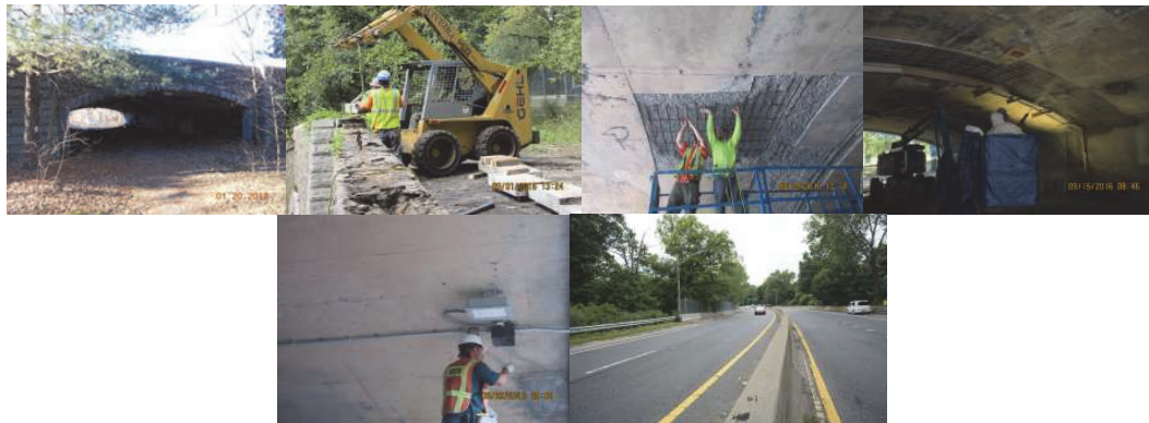
Mosholu Parkway Bridge over Equestrian Path. (Credit: NYSDOT) Bridge Before, During (Removing Stones and Stone Masonry, Removal and Repair of Deteriorated and Unsound Concrete, Repairing the Underdeck Lighting), and After Construction.
