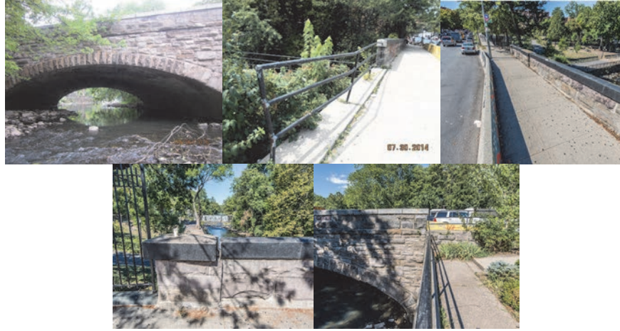
East 180 th Street Bridge over Bronx River Before Construction. Elevation Right in September 2016. July 2014: Bent Railing at Side Approach. (Credit: NYSDOT) West View and the North and South Parapet Walls.
