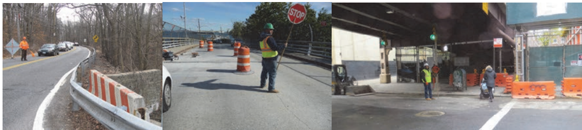
Flagperson at the Rockland Avenue at Manor Road Culvert, Hannah Street Over SIRT, and at the Queensboro Bridge Ramp to East 62 nd Street From Queens.
