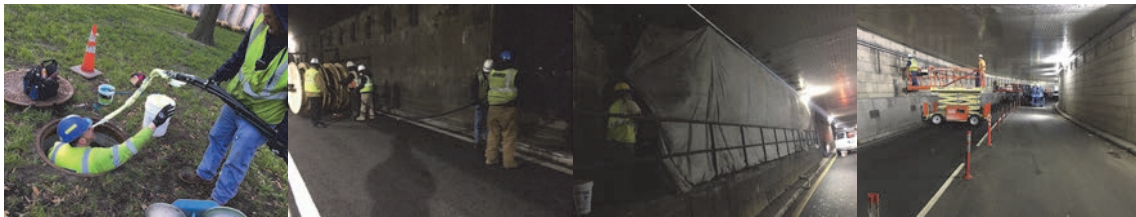
April 2016 - Installing Cables. July 2016: Painting Standpipe in the Southbound Battery Park Underpass. August 2016: Installing Conduits in the West Street Underpass.
