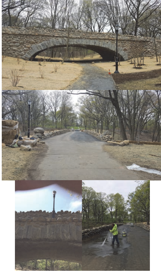
April 2017 - at Substantial Completion. New Light Pole on Bridge. May 2017 – Power Washing the Road Surface.
