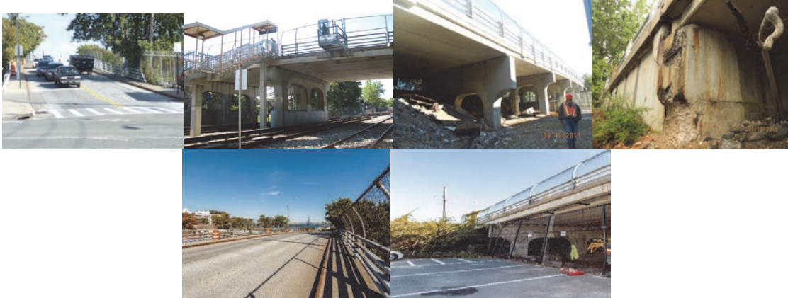
Hannah Street Bridge Over SIRT South Shore. Spans 1-4 - Right Elevation. October 2015: Large Deep Spall on Right Corner of Beginning Abutment. (Credit: NYSDOT) Before Construction.
