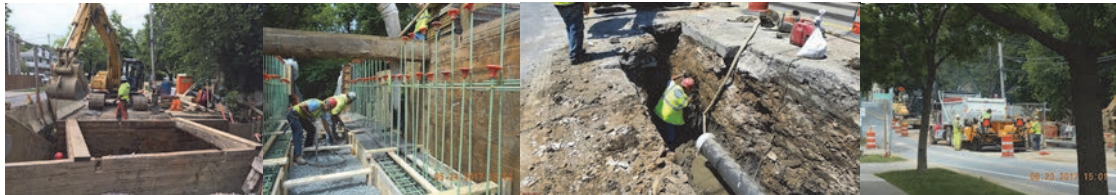
May 2017 - Looking West - Installing Shoring Around Excavation. Looking North - Placing Concrete for Footing. June 2017 - . Looking Down and Northwest Along Forest Avenue - Installing the New 12 Inch Water Main. Looking Northwest - Placing Temporary Asphalt Over 12 Inch Water Main Trench on Forest Avenue.
