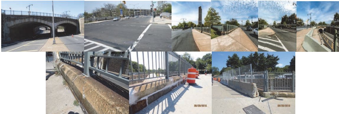
Southern Boulevard Bridge over East Fordham Road Before Construction. West Side, East Side, Eastbound Roadway, and Missing Section of Fence. August 2016: Cracked Cap Stone at Right Wingwall. Repaired Joints on Right Parapet. Jersey Barriers and Fence Above the Deck on Span 1.
