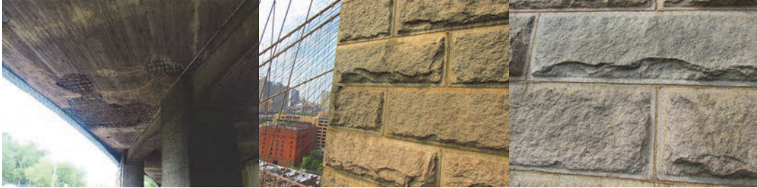
Hollow Sounding And Delaminated Concrete Areas With Exposed Rebars on the Sunrise Highway Bridge Westbound over Laurelton Parkway in 2014. Brooklyn Bridge Tower Stone Delamination in 2016.
