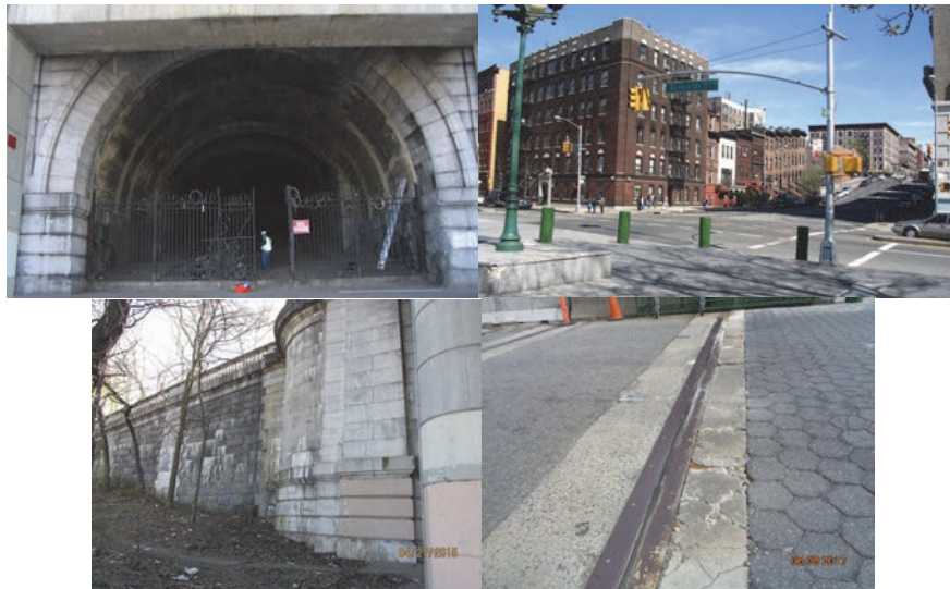
Riverside Drive Bridge over West 145 th Street. April 2015: East Abutment Wingwall. April 2017: Top of Deck, at Entrance to Riverbank State Park. (Credit: NYSDOT)
