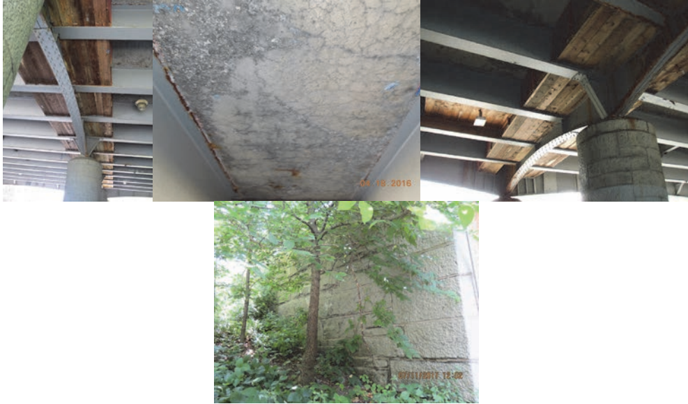
June 2015: Span 1 Deck – Hollow Sounding Concrete Areas are Covered by Timber Planks That are in Good Condition. April 2016: Span 2, Underside of Deck, Bay 3 - Exhibits Scaling, Mapcracking with Localized Efflorescence, and Dampness Over Approximately 50%-60% of its Surface. (Credit: NYSDOT) July 2016: Span 2 Timber Shielding. July 2017: Cladding on the Left Side of the End Abutment in Good Condition.
