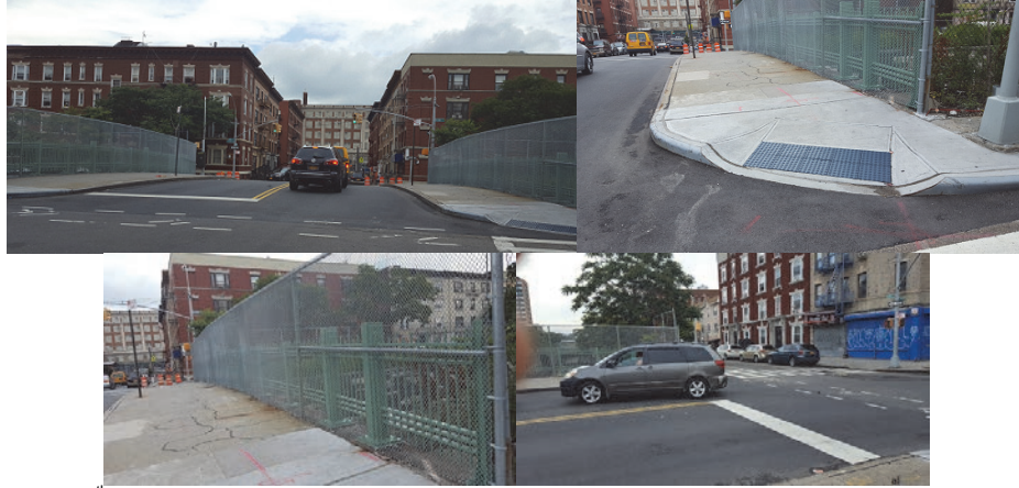
East 187 th Street Bridge over Metro North After Construction – Asphalt Overlay. Southwest Pedestrian Crosswalk. New Chainlink Fence. North View.
