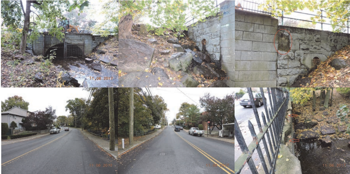
Forest Avenue Bridge Over Clove Lakes Park Stream. November 2017: Right Elevation at Upstream. Beginning Abutment Right Wingwall. End Abutment Stone Masonry Wingwall. Beginning and End Approaches. Right Side Parapet and Concrete Coping. (Credit: NYSDOT)
