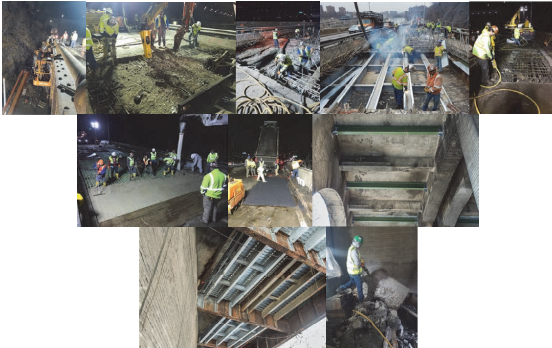
March 2017. Deck Removal During Northbound Repairs. Concrete Placement for Full-Depth Deck. Asphalt Placement Over Cured Deck. April 2017: Newly Installed Steel Angles Under Span 38, and Steel Installed Above the Harlem River Drive.
