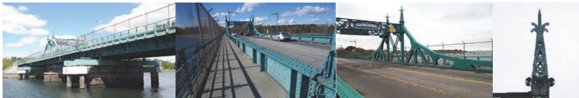
City Island Road Bridge in 2010. (Credit: Bojidar Yanev) Span 4, Right Sidewalk Near Pier 4 in October 2013. Vertical Clearance Posting. (Credit: NYSDOT) 9 Foot Tall Ornamental Finial.
