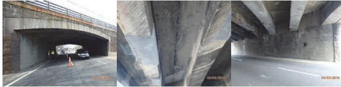
Douglaston Parkway Bridge Southbound Over Cross Island Parkway. March 2016: Right Elevation. Span 1 Concrete Beams Exhibit Spalls With Exposed Rebar Which Are Covered by Wire-Mesh Netting. (Credit: NYSDOT)
