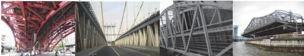
Brooklyn Bridge Franklin Square Truss. General view of Manhattan Bridge Trusses B and C From the Lower Roadway on the Main Span. (Credit: NYSDOT) Chambers Street Pedestrian Bridge Truss. Madison Avenue Bridge Truss Swinging. (Credit: NYSDOT)
