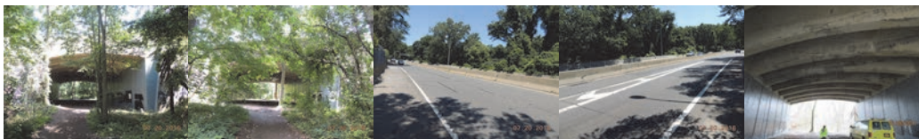
Elevation Left and Right, and Approach Begin and End in July 2016. (2016 Credit: NYSDOT) January 2017: Span 1 Under Girders Looking North.
