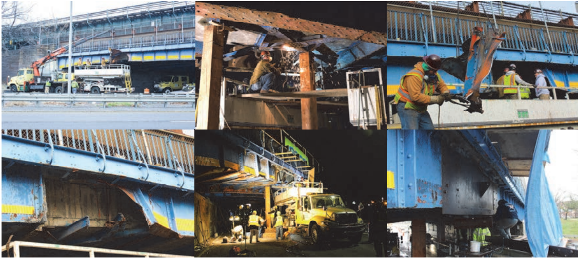
On January 9, 2016, a Truck Travelling South on the Parkway Struck the Bridge, Causing Damage to a Fascia Girder and its Preceding Girders, Stringers, and the Hanging Bars of a Strongback. Crews Responded, Cut a Portion of the Sheared Girder and Spliced it With a New Section and Installed Shoring.
