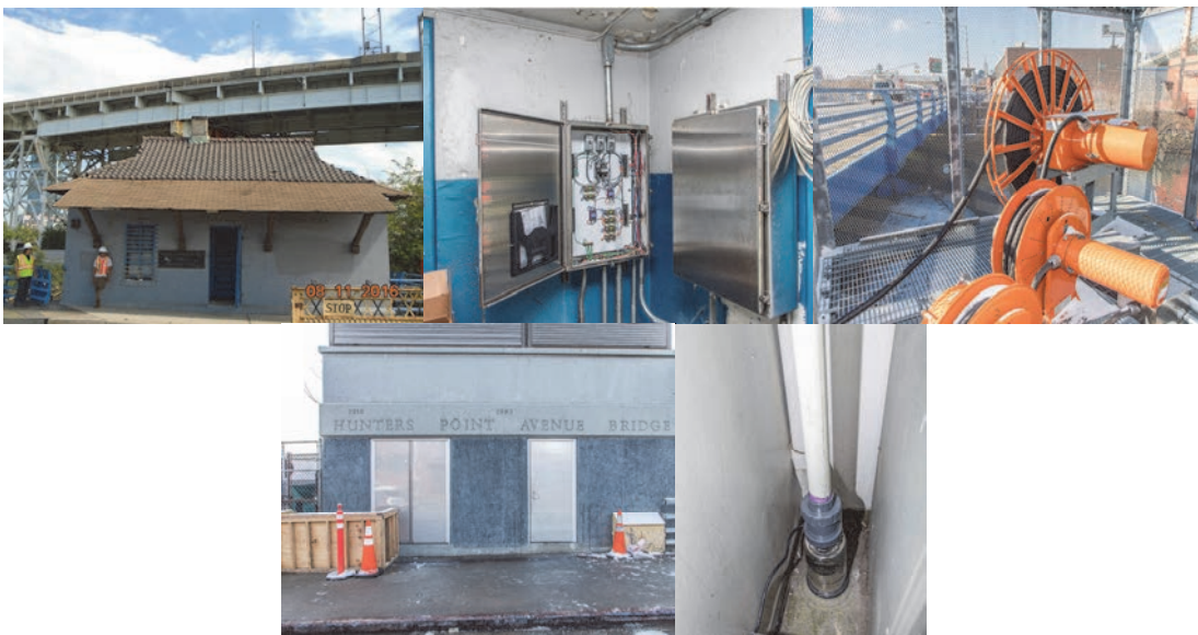
2016: Borden Avenue Bridge Operator House. 2017: Borden Avenue Bridge Traffic Panel. Submarine Cables. 2017: Hunters Point Avenue Bridge New Double Doors. Sump Pump and PVC Pipe.
