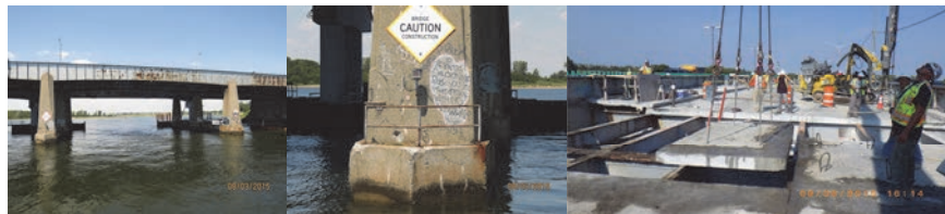
Old Gerritsen Inlet Bridge in August 2015 - Span 6, Right Fascia, Looking Left. Span 6, Pier 5, Column 3 – Construction Sign and Non-Functioning Light. (Credit: NYSDOT) September 2015: Removing Saw-Cut Deck Panels.
