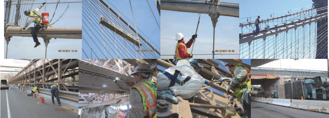
Brooklyn Bridge Contract #6 in 2014 - Painting Main Cables and Suspension Ropes. Painting at Main Bridge – Safety Barrier and Touchup. Containment at Ramp A, Span 4.
