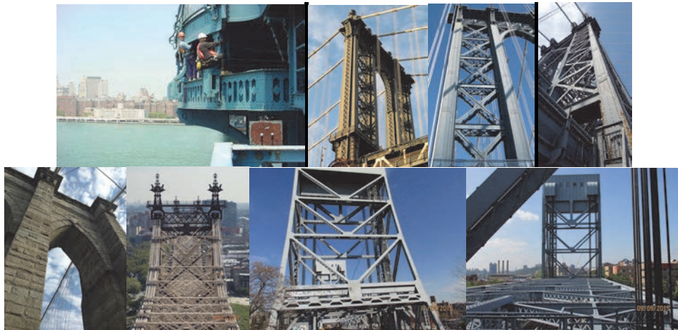
Inspectors on Manhattan Bridge Tower. (Inspector Credit: NYSDOT) Manhattan Bridge Tower. (Credit: Michele N. Vulcan) Manhattan Bridge Tower Detail. (Credit: Russell Holcomb) Williamsburg Tower Detail. (Credit: Bojidar Yanev) Brooklyn Bridge Tower. (Credit: Earlene Powell) Ed Koch - Queensboro Bridge Tower Top. Broadway Bridge Begin and End South Tower Face. (Credit: NYSDOT)
