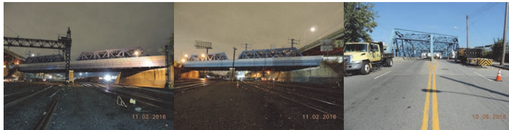
East 149 th Street Bridge over Amtrak – CSX. November 2016: Elevation Left and Right. Beginning Approach. (Credit: NYSDOT)
