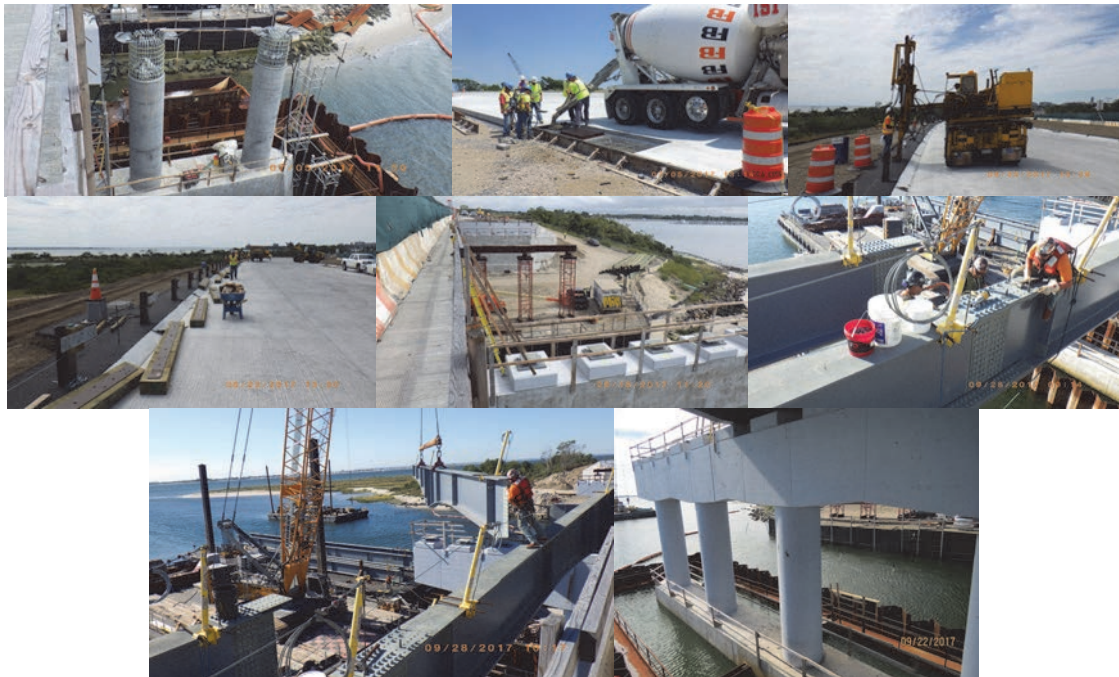
Gerritsen Inlet July 2017: Pier #2 - Plinth and Columns Completed Prior to Cap Beam Installation. Placing P.C.C. Pavement in Approach Roadway Block Out for Catch Basin Frame and Grate. August 2017: Driving Steel Posts for Steel-Backed Timber Guide Rail at Asphalt Shoulder of Approach Pavement. Installing the Rail. September 2017: East Abutment at Top. Pier #2 With Bearings In Foreground, and Temporary Support Between Pier #2 and the East Abutment, Prior To Delivery Of Eastbound Steel Girders. Iron Workers Bolting up Girder Splice at Pier #2 on The Eastbound Side Of the Bridge. Girder Being Lowered Onto Pier #2 and Temporary Support. Pier #1 – New Pier Wall. (Pier#1 Credit: NYSDOT)
