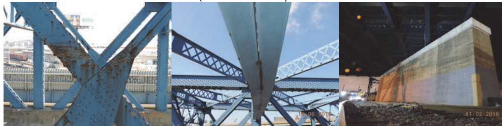
Span 2, Truss T2 - Left Face of the Gusset Plate and Adjacent Diagonal Member Exhibit Scrape Marks and Paint Loss With Minor Surface Corrosion Due to Vehicular Impact. Span 1, Sway Strut Bracing Between Truss T2 and T3 - Brace Bottom Flange Exhibits Bending Toward Span 2 due to Vehicular Impact. Pier 1. (Credit: NYSDOT)
