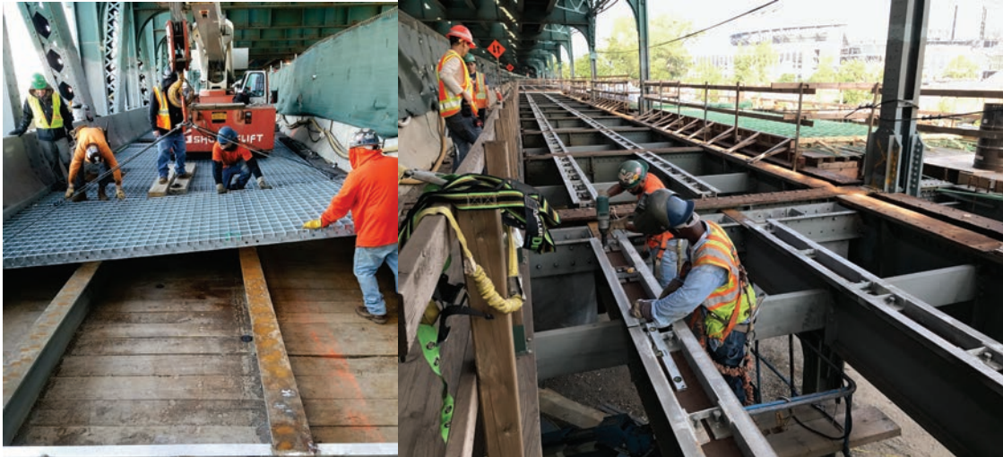
Contractors Installing the New Bascule Span Grid Deck on the Roosevelt Avenue Bridge in Flushing in March 2017. The Bridge is Permanently Set in a Closed Position Since the Late 1950's. Installing Haunch Angles at the West Viaduct Roadway Deck in July 2017.
