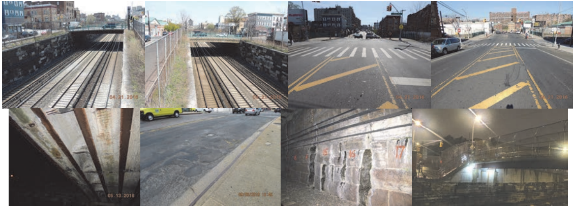
East 180 th Street Bridge: April 2016 - Left and Right Elevations. Beginning and End Approaches. May 2016: Diaphragms in Bay 2 Exhibit Underside Spalling With Exposed, Debonded Rebar. (Credit: NYSDOT) September 2016: The Left Side of the Roadway Looking Toward the Beginning Abutment - The Wearing Surface Exhibits an Uneven Surface, Map Cracking and Small Potholes. February 2017: End Abutment Looking Northeast. Water Leakage Stains on the Bottom Portion of the Stem. Night View.
