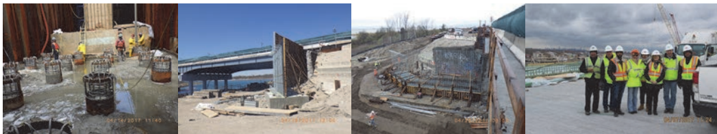
Gerritsen Inlet April 2017: Pier #1 Cofferdam. Pumping Concrete Into Steel Pipe Piles. New Pier #1 Footing and Plinth From Previous Stage Show in Background. East Abutment Footing With Rebars and Formwork for Abutment Wall. Stage 3 Completed Bridge is in the Background. West Abutment Forms and Rebars in Place for Footing. Concrete Abutment Wall Rebar Placement in Progress. Site Visit – Assistant Civil Engineers Khalid Mohammed, Yuriy Kheyman, and Juan Medina-Yan, Associate Project Manager Alina Platonova, Community Associate Shahnaz Begum, Associate Staff Analyst Vera Ribakove, Administrative Engineer Daniel Hom, and Civil Engineer Chetan Patel – (Credit: Eric Callender)
