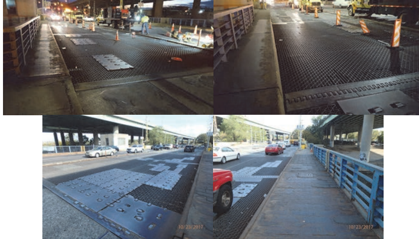
January 2017: Bridge Grating. October 2017: Span 9, Right Side, Eastbound Travel Lanes. The Top of the Steel Open Grid Deck has Multiple Steel Plates Installed Throughout the Eastbound Lanes to Cover the Damaged Areas of the Gratings. Span 9 Right Sidewalk. (Credit: NYSDOT)
