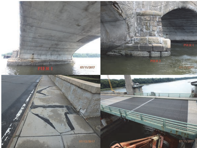
July 2017: Pier 1 Begin Face. Pier 2, Left End of Pier Nose - Typical Mortar Loss Between Stones. Span 6 Right Sidewalk Exhibits Full Width Shallow Spalls – Partially Patched by With Asphalt. Top of Span 4. (Credit: NYSDOT)
