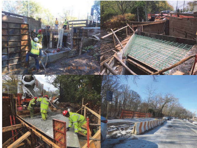
October 2017 – West Walls and Wingwalls Formwork. Looking West - Formwork and Rebar for the Roof Slab. Placing Concrete for the Roof Slab. Sidewalk.
