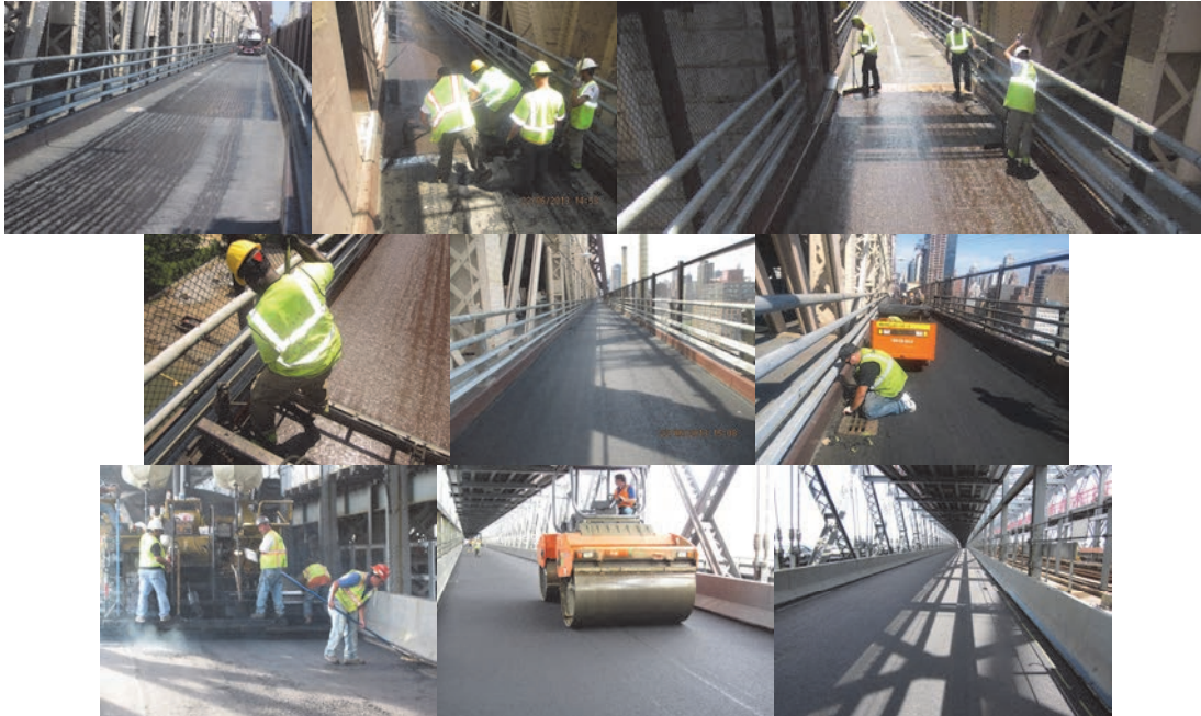
Repairing the Concrete Overlay on the South Upper Roadway of the Ed Koch – Queensboro Bridge in June 2013. (Credit: Sunil Desai) Repaving the Williamsburg Bridge in 2011.
