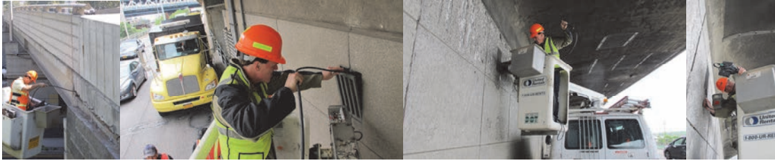
Director of Bridge Management Kevin McNulty Inspecting the Bridge Carrying the Belt Parkway over Ocean Parkway, Utilizing the Unit's Borescope. June 2015: Inspecting the Brooklyn-Queens Expressway Between Cadman Plaza and Atlantic Avenue.
