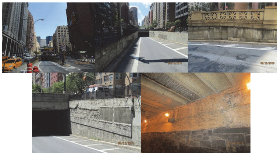
Park Avenue Tunnel – Left and Right Elevations in 2016. Begin Left Wingwall - Stones are Partially Dislodged, Cracked and With Missing Mortar. End Right Wingwall - Wall is Spalled and Exhibits Hollow Concrete Areas That are Shielded With Wire Mesh. End Abutment (Near South Portal) – Bricks Exhibit Deteriorated Mortar. (Credit: NYSDOT)
