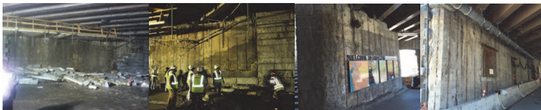
Prospect Street East Abutment Collapse in July 2014. Washington Street East Abutment.
