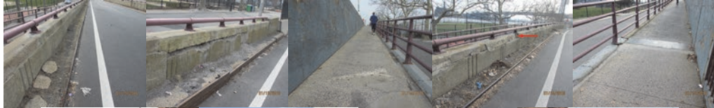
January 2016: South Approach Ramp - Span 2, Left Side Safety Walk and Curb. End Approach, Left Parapet. Span 4, Left Cantilever Sidewalk. North Approach Ramp – Span 2, Right Parapet and Safety Walk. Span 3, Right Cantilever Sidewalk. Elevation Right. 2016: Main Bridge – Spans 1 and 2 at Left Side. South and North Approach Ramps, Span 1 Top of Deck Wearing Surface.
