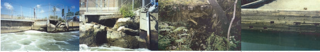
From Study of the FDR Drive: Location #2 – Damaged Seawall at Segment #5. Sinkhole at Location #6 at East 59 th Street. From Study of Carroll Street Bridge: General View of the Southwest Crib Wall With the Delamination of the Timber Stretchers in the Tidal Zone.
