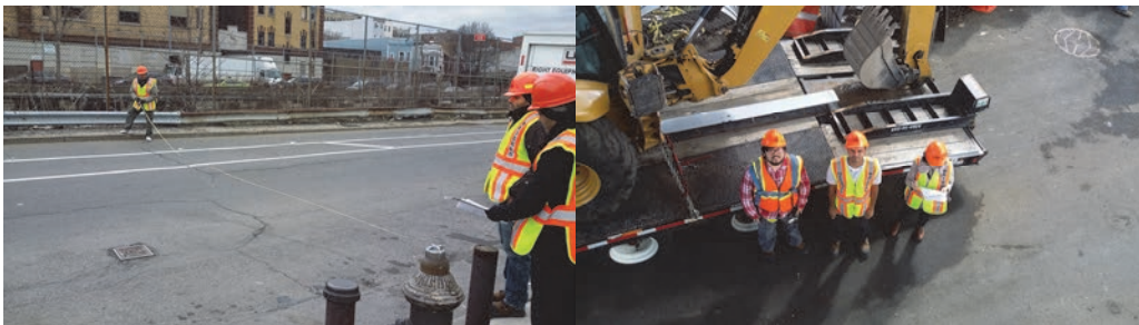
January 2017: Inspecting the East 180 th Street Bridge over Metro North – Assistant Civil Engineer Arif Hussain, and Civil Engineers Vishal Jariwala and Ruchit Patel. (Credit: Scott Alnwick) June 2017: Inspecting the Boston Road Bridge over Hutchinson River – Civil Engineering Intern Edward Shao, Civil Engineer Vishal Jariwala, and Assistant Civil Engineer Olga Goranova-Rouyne. (Credit: Krzysztof Lamczak)
