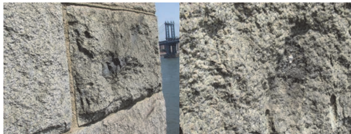
Brooklyn Bridge Tower Stone Scaling in 2016.
