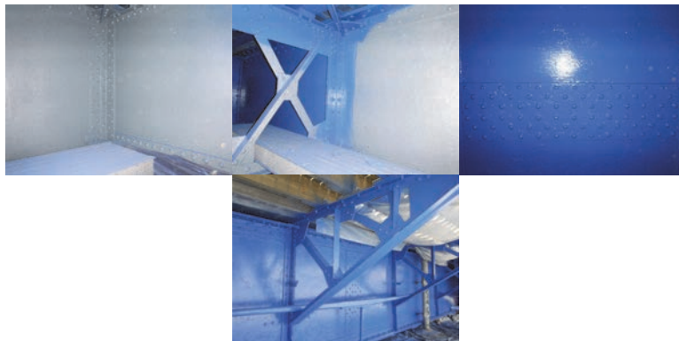
Movable Bridge Preventive Maintenance Contractor Removing Paint and Repainting on the Borden Avenue Bridge.
