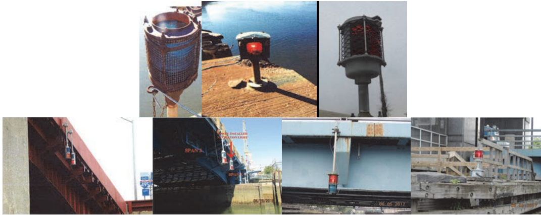
Northern Boulevard Bridge - Bridge and Pier Marine Navigational Lighting. Grand Street Bridge- Left Side Channel Light. Pulaski Bridge - Center Lights at Span #26. Third Street Bridge - Span #3. Ninth Street Span 2 Right Fascia and End Left Channel Embankment. (Credit Grand, Third, and Ninth Street: NYSDOT)
