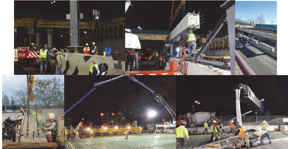
April 2017: Stage 3 - Erection of New Steel Columns and Pier Caps at the Center Pier. Alignment of Final Hollow Slab Unit for Stage 3. May 2017: Concrete Placement for Stage 3 Bridge Deck. June 2017: Concrete Placement for South Sidewalk and Median.
