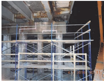
Mill Basin Bridge Scaffold Used During Pier Cap and Pier Column Repairs.
