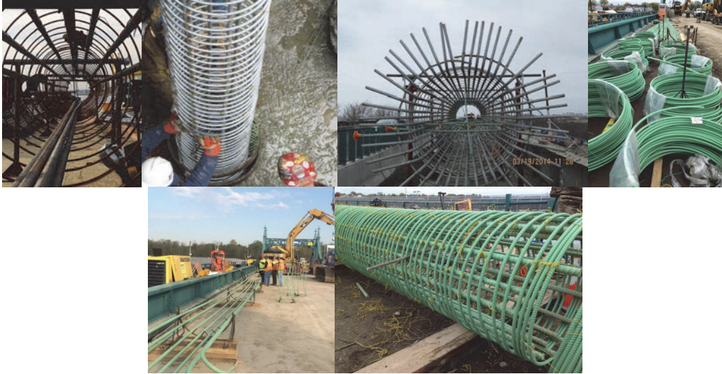
City Island, Gerittsen Inlet, and Bay Ridge Avenue Bridge Rebar Cages. 2016: Rebar Cage Assembly for the City Island Bridge. May 2016: Each Drilled Shaft Requires a Custom-Built Rebar Cage. These Steel Structures Strengthen the Concrete That is Placed Within Each Shaft Casing. Steel Bars are Laid Out on a Template to Form the Shape of the Cage, and are Then Tied Together. Once completed, the cage is Lifted by Crane and Placed Within a Corresponding Drilled Shaft.
