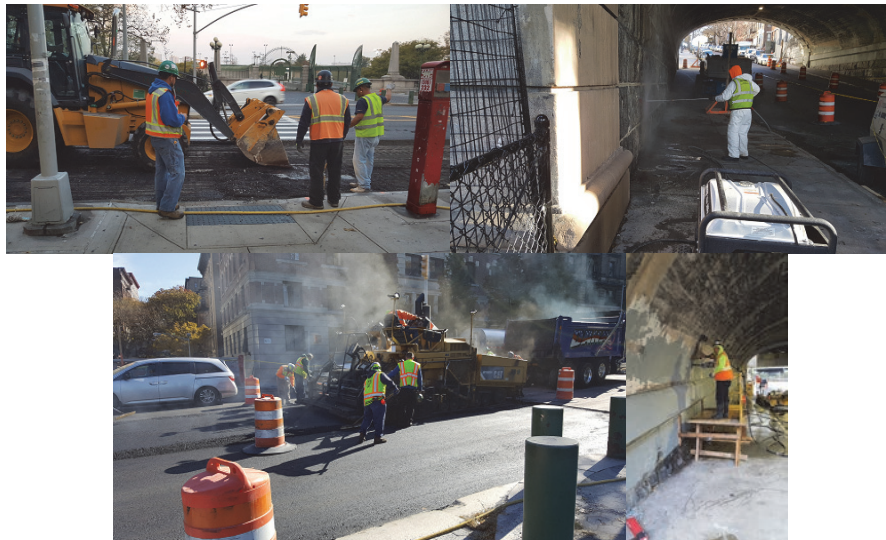
Riverside Drive Bridge over West 138 th Street During Construction – Asphalt Milling, Power Washing, Asphalt Placement, and Weep Hole Drilling.
