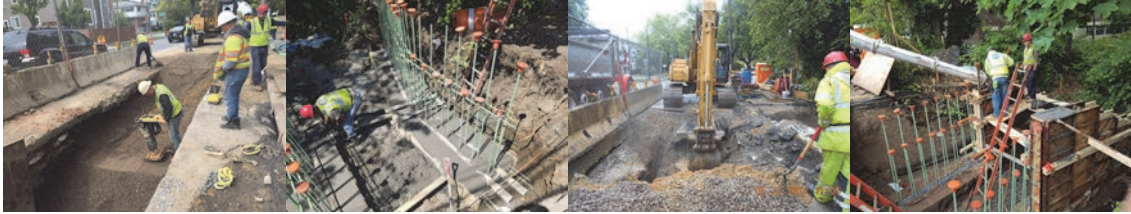
Forest Avenue Culvert over Randall Avenue in May 2017 - Looking West. Backfilling the Trench Over the New 20 Inch Iron Pipe Water Main. Looking South - Placing Rebar for Wingwall Footing. Looking West - Excavating and Removing the Old Culvert. Looking Northwest. Placing Concrete Into Formwork for the Wingwalls.
