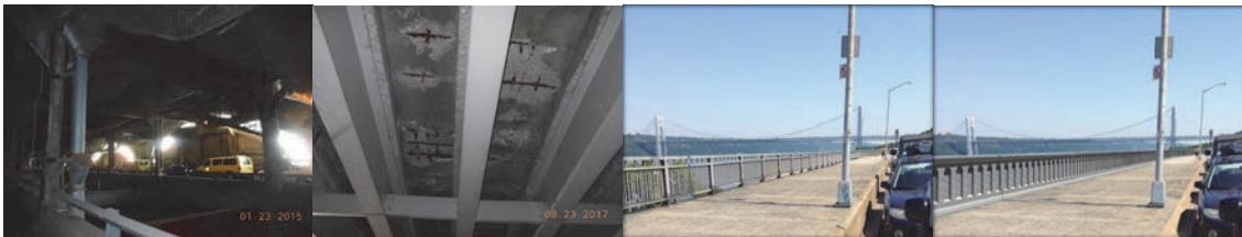
2015: Underside of Span 30, Looking Southwest (NYCDOT Maintenance Garage Area). 2017: Span 5 Underside of Deck Bays 16 and 17 - Spalls With Exposed Rebar. (Credit: NYSDOT) Current and Proposed Bridge Railing.
