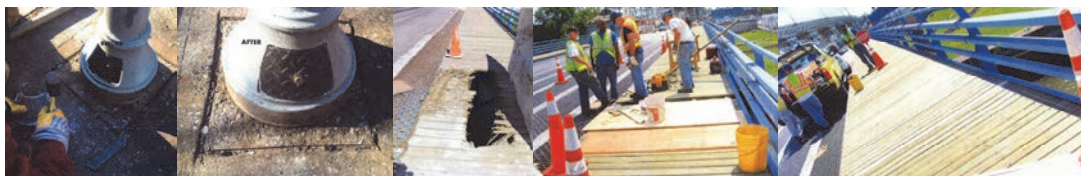
East 14 th Street Bridge Over LIRR Bay Ridge –Ironworkers Fabricated and Installed the Bottom Cover of the Ventilation Post on the Right Sidewalk. June 2017 Safety Flag: Borden Avenue Bridge over Dutch Kills – Broken Wooden Planks of the Right Sidewalk at Span #1.
