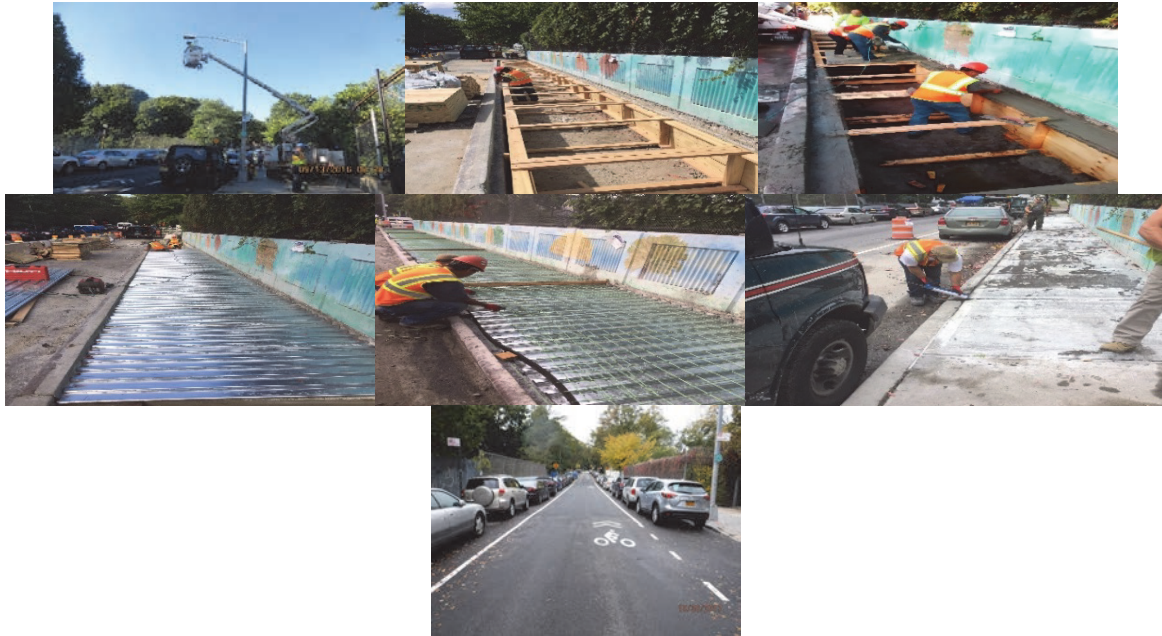
80 th Road Bridge Under Construction. October 2017: End Approach Pavement and Spans 1 to 3 Wearing Surface Repaved With Asphalt Concrete. (October Credit: NYSDOT)
