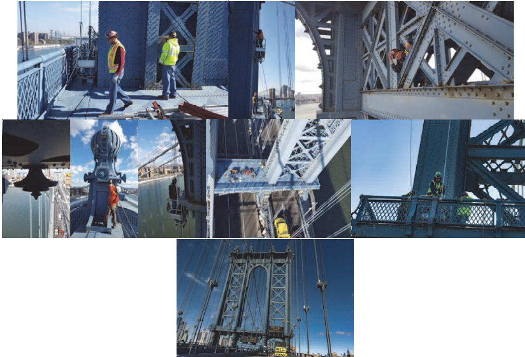
Ornaments on the Manhattan Bridge Towers Were Flagged as Potentially Hazardous and Removed by In-House Ironworkers in October and November 2016. (Credit: Bojidar Yanev) Using Spider to Remove Ornament at Cable C West in 2016. (Credit: Samuel Teaw)
