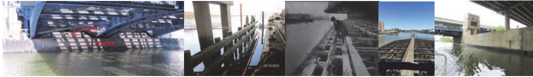
Metropolitan Avenue Bridge Fender. Installing the Fresh Creek Bridge Fender System in 2013. Inspecting a Damaged 145 th Street Bridge Fender in 1917. North Fender Pier of 145 th Street Bridge in 2015. (Credit: Lity Barreto) Unionport Pier 8 Fender.
