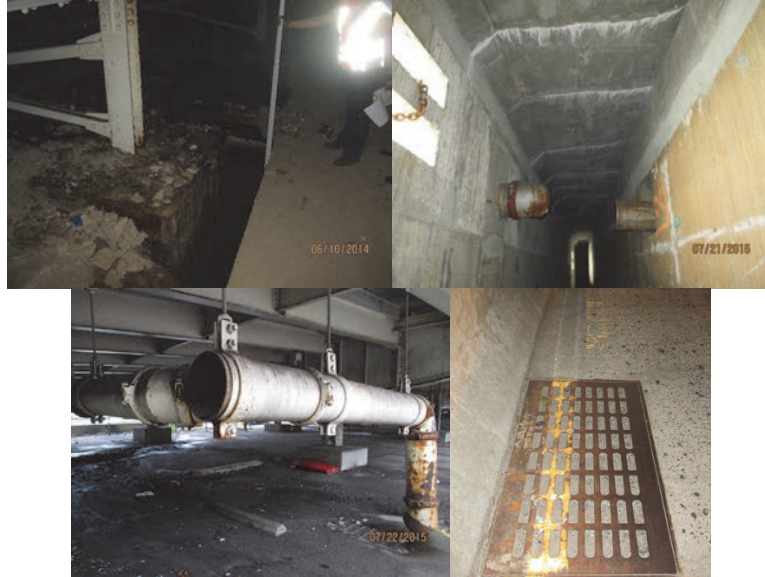
Scour Hole at Pier #3 in 2014. 2015: Span 5 – Right side. Span 46 – Left Side. Downspout Near North Abutment. (Credit: NYSDOT) Typical Clogged Scupper Inlet.
