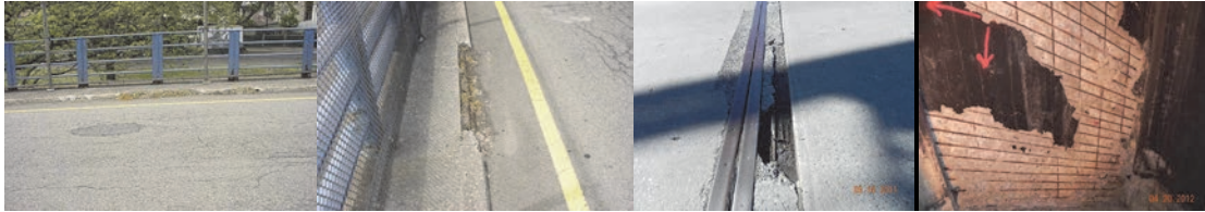
Spalled Section of Curb on the East 8 th Street Bridge in 2006. (Credit: NYSDOT) Spalling With Exposed Rebar on the Beginning Abutment Joint Header of the Westchester Avenue Bridge over the Bronx River in 2011. Underdeck Spalling With Exposed Rebar on the Concourse Village Avenue Bridge over Metro North in 2012.
