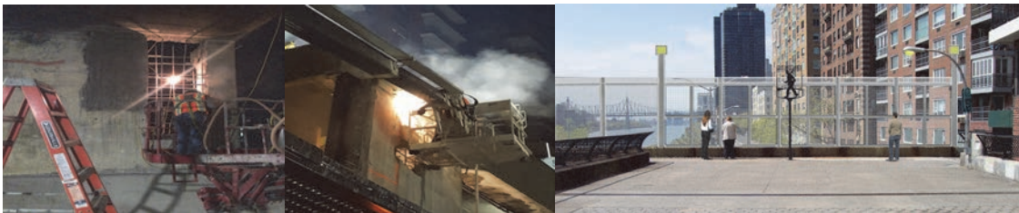
Retrofitting the North Abutment (8 Months). Rendering of the Viewing Window at the Southern Terminus of the John Finley Walk. (Credit: NYCDDC)
