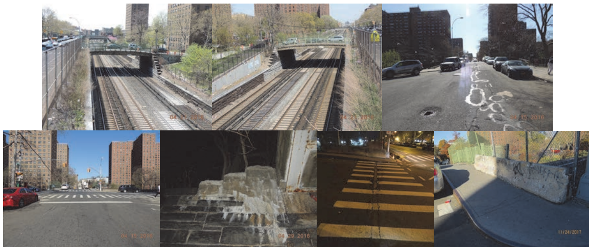
East 169 th Street Bridge: April 2016 - Left and Right Elevations. Beginning and End Approaches. Moderate Map Cracking With Efflorescence in the Reinforced Concrete at the Top of the Beginning Right Wingwall. (Credit: NYSDOT) February 2017: End Abutment, Joint with Deck. Full Length Cracks With Deteriorated Wearing Surface. November 2017: Left Sidewalk Near End Abutment - Temporary Jersey Barrier in Place.
