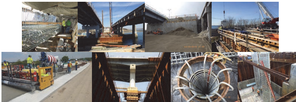
Gerritsen Inlet February 2016: Galvanized Rebars in Place for East Abutment Footing. March 2016: Driving 24" Diameter Steel Shell Piles at Extension of Pier #1 Cofferdam. New Westbound Bridge at Left. Existing Eastbound Bridge at Right. April 2016: Completed Portion of New East Abutment of the Bridge. New Bridge at Left. Placing Concrete at West Abutment Back Wall With a Crane and Bucket. May 2016: Placing and Finishing On-Grade Pavement at Approach. Cofferdam at Pier #2. Column, Pier Cap and Structural Steel Placed in Stage 1. June 2016: Rebar Cage Placed Inside Steel Pipe Pile Prior to Concrete Operation. Lowering Column Rebar Cage Onto Footing Rebars at Pier # 2.
