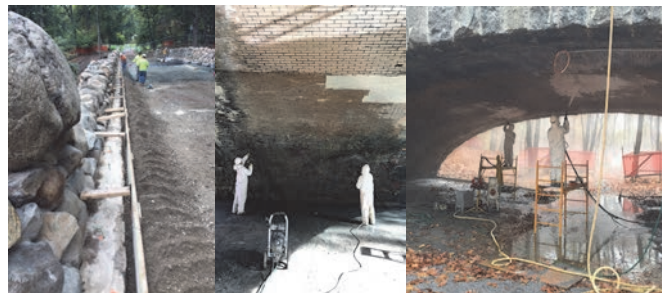
October 2016: Concrete Curb Layout. November 2016: Cleaning the Bricks Under the Bridge Arch. December 2016: Cleaning the Historic Stone Masonry and Removing Graffiti.
