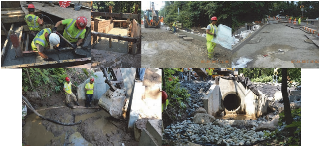
June 2017 – Pouring Manhole Walls. July 2017 – Placement of Low Strength Concrete Complete. Placement of Concrete Curb Along the South Gutter Line. Placing Roadway Base. Excavation of Material on Top and in Front of the Apron Slab. Placement of River Bed Stones, Medium Stones, and Boulders Adjacent to the Culvert Walls and Apron Slab.
