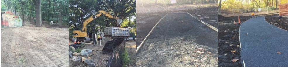
August 2016: North and South of Bridge – Clearing and Grubbing. November 2016 Placing Granular Fill Material (Crushed Stone) on the Bridge Pathway Under the Bridge Arch.
