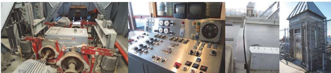
Non-operational Span Drive Machinery. Current Operator Desk and Bronx Approach End Dam. Gate House.
