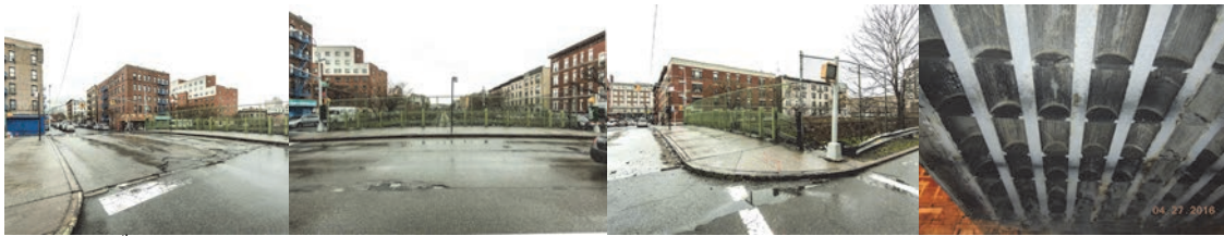
East 187 th Street Bridge over Metro North Before Construction - Southeast and North Views. Southwest Crosswalk. April 2016: Span 1, Underside of Deck Exhibited Minor Mapcracking and Efflorescence. (Credit: NYSDOT)
