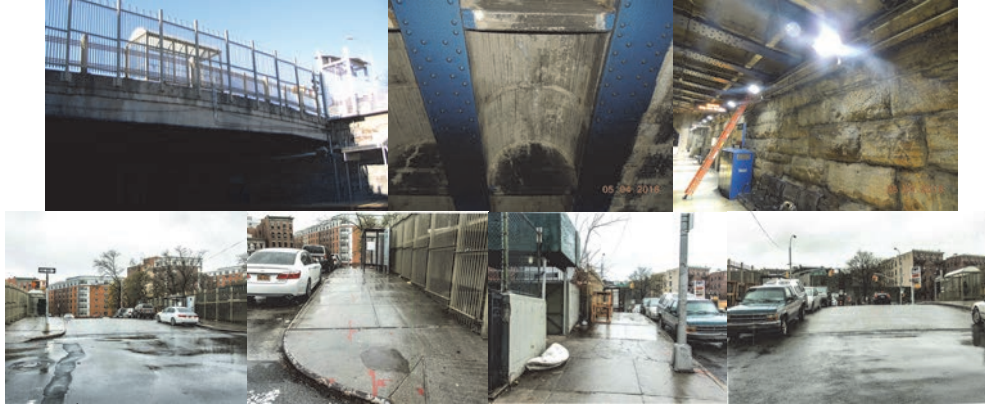
East 162 nd Street Bridge over Metro North Before Construction. May 2016: Span 1, Underside of Deck Exhibits Longitudinal Cracks With Efflorescence. End Abutment Stem. (Credit: NYSDOT) Northeast Side. Southwest Pedestrian Crossing. North Sidewalk. East View.
