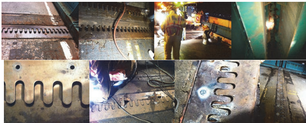
July 2013 PIA Safety Flag on the old City Island Bridge. The repairs, conducted after a record-breaking heat wave, involved opening the joint plates and installing plug welds, which helped correct the plates' position and recreated the proper gap to allow the bridge to expand and contract safely. Finger Joint Before the Repair. Open Finger Joint. Division Crews Repairing the Joints. View Beneath the Finger Joint. The Joint Plates are Placed to Check for the Proper Gap. Leveling the Plate Before Welding. Close-Up of a Plug Weld. After 17 Plug Welds, the Finger Joints Sit Flush on the Roadway.
