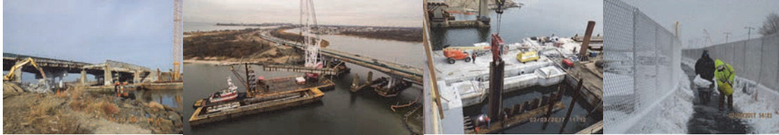
Gerritsen Inlet January 2017: Final Demolition of the West Abutment During Stage 3. Barge-Mounted Crane at Right in Process of Removing the Last Sections of Structural Steel From the Old Bridge. The Last Structural Steel Section of the Bridge Being Lowered Into a Barge for Removal From the Site. February 2017: Driving Sheet Piles for the New Bridge Pier #1 Cofferdam. Old Pier #4 After Columns Were Removed is Visible East of New Cofferdam. Clearing and Maintaining the Pedestrian/Bicycle Path in the Vicinity of the Bridge After the February 9 Snow Storm.
