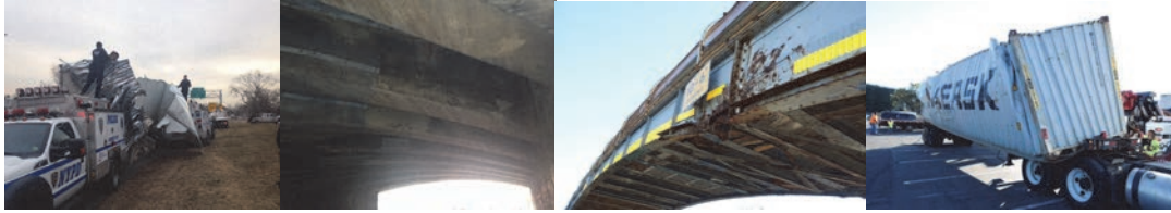
Douglaston Parkway Bridge Strike in 2015: Police Observing the Truck Damage. Underside of Bridge Concrete Beams Only Exhibited Scratches. (Credit: Artemio Angeles) 17 th Avenue Pedestrian Bridge Strike in 2015.
