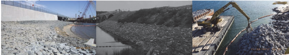
Riprap Installed in 2013 on South Side of Belt Parkway Bridge over Fresh Creek, Facing East. Riprap at the Southwest Side of the South Approach of the Shore Road Bridge over Hutchinson River in 1908. Barge-Mounted Crane Placing Riprap Stones on the South Slope of Gerritsen Inlet at the West Abutment in 2017.
