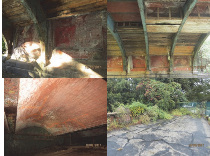
Pier 1 Solid Stem Wall Between Bays 4 and 5 – the Lower Portion of the Pier End Face (Below the Timber Shielding) Exhibits Efflorescence, Dampness and Leakage Over a Large Area. Span 2, Underside General View. Span 2, Underside Brick Arch at Girder Near Pier 2 Exhibits Efflorescence over Most of the Surface Area. Span 3, Left Parapet and Railing Interior Face. (Credit: NYSDOT)
