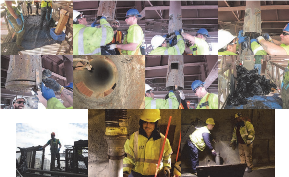
Preventive Maintenance Contractors on Traveler #3 South on the Ed Koch – Queensboro Bridge Conducting Drainage Cleaning. Drain Crew: Highway Repairer Anthony Irizarry, Supervisor Highway Repairer Michael Parise, and Assistant City Highway Repairer Giavonni Caballero. (Crew Credit: James Campbell)
