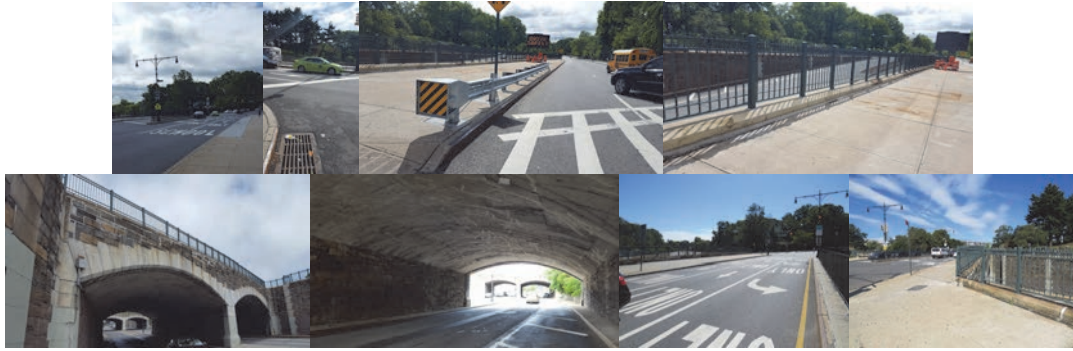
Southern Boulevard Bridge After Construction - New Asphalt at West Side and at the Eastbound Roadway. New Guiderail and Fence. Section of Fence. Repaired Joints at Fascia. Sealed Crack and Installed Weep Holes at Westbound Fordham Road. September 2017: Barriers Removed After Construction – Top of Span 2 Looking East. Top of Deck at Beginning Approach Looking West.
