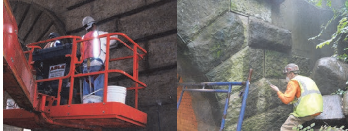
Pointing Joints on the East Face of the Brooklyn Anchorage of the Manhattan Bridge. Pointing the Masonry on the East Drive Bridge (East Wood Arch).
