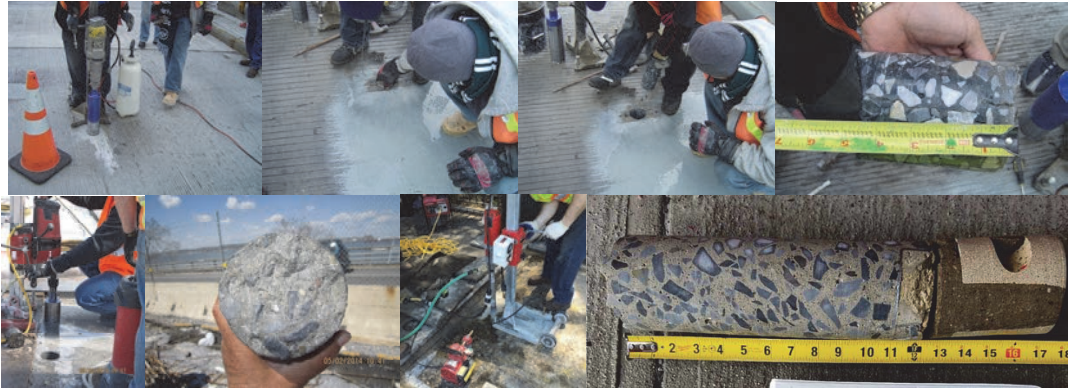
Removing a Core From 252 nd Street Bridge over Henry Hudson Parkway in January 2009. (Credit: Masroor Mahmood) Core Sampling on the Bay Ridge Avenue Bridge in 2014. Utilizing a Coring Machine to Obtain a Concrete Core for Testing in June 2016 from the Westbound BQE over Adams Street.
