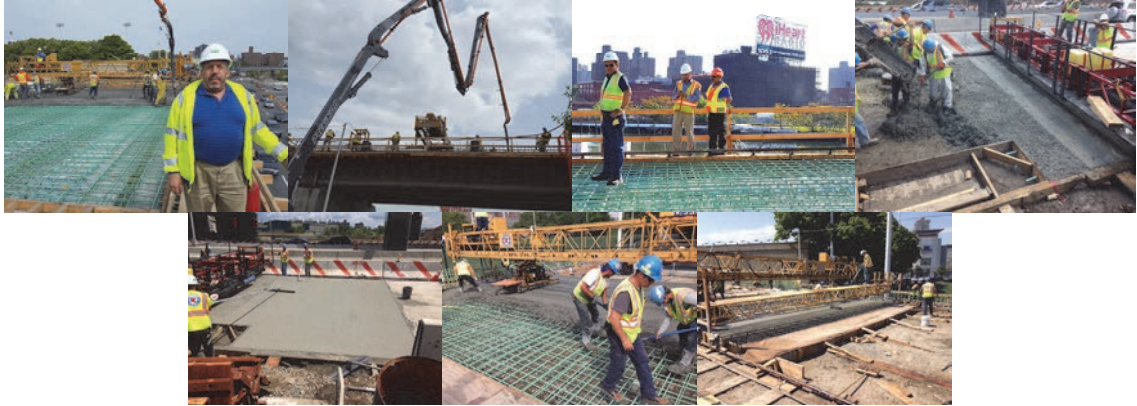
May 2017: Associate Project Manager Richard Solomon Observing the Placing of Concrete for the Southbound Bridge Deck Spans 6-7. (Credit: Salome Stulberg) May 2017: Associate Project Manager Artemio Angeles (in foreground), Division Quality Assurance Assistant Civil Engineer Syed Naqvi Bridges, and NYSDOT Representative Yogesh Chokshi. (Credit: Richard Solomon) PCC Pavement at Southbound South Approach. June 2017: Contractors Utilizing a Bidwell Bridge Paver for the Southbound Bridge Deck. (Credit: Richard Solomon)
