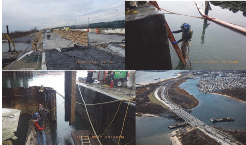
December 2017: Wood Forms Erected on the Bridge for the Future Concrete Barrier Separating the Pedestrian/Bicycle Walkway from the Future Eastbound Belt Parkway Traffic. Pedestrian Fence Anchor Bolts at Left. Diver at Pier # 2 Entering the Waterway to Cut the Steel Cofferdam Sheeting Prior to Removal. Removing Steel Sheeting Cut from Cofferdam #2. Gerritsen Inlet Bridge in December 2017.
