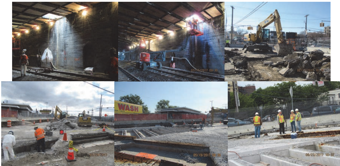
January 2017: Shielding Installation Below the Bridge Deck and Above the Railroad Tracks. Debris Removal Through Protective Shielding. February 2017: Stage 1 Demolition of Pavement and Concrete Overlays. March and May 2017: Stage 1 Demolition of Concrete Bridge Deck and Beam Encasements. May 2017: Site Visit – Assistant Civil Engineer Daniel Smith, Deputy Commissioner Robert Collyer, Community Liaison Nancy Catapano, and Resident Engineer Joe Catapano.
