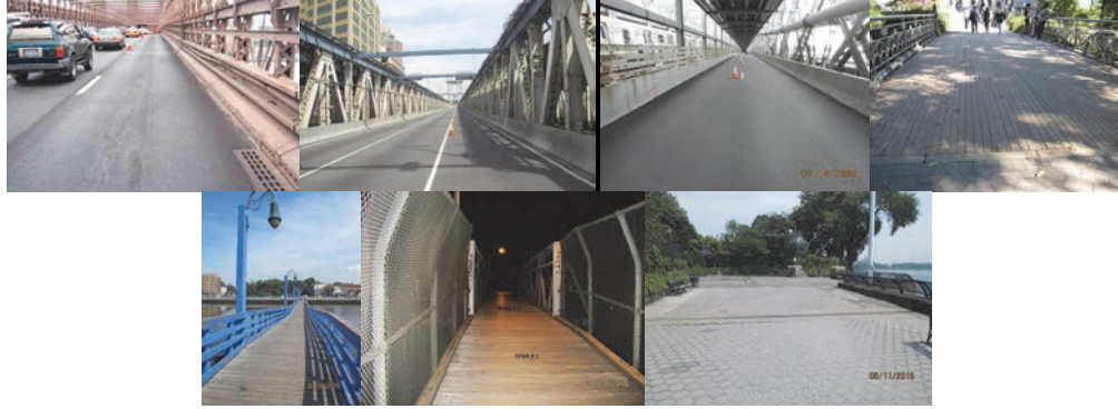
Brooklyn Bridge Wearing Surface. Manhattan Bridge Wearing Surface and Safety-Shaped Barriers. Williamsburg Bridge South Inner Roadway Wearing Surface. (Credit: NYSDOT) West 86 th Street Pedestrian Bridge (Southwest Reservoir Bridge) Wooden Wearing Surface. Ocean Avenue Pedestrian Bridge over Sheepshead Bay. 60 th Road Pedestrian Bridge over LIRR. Promenade over FDR Drive Span 43. (FDR Credit: NYSDOT)
