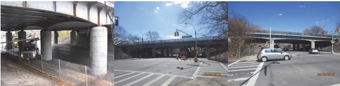
Nostrand Avenue Bridge Pier 1 and 2 Columns in December 2014. Left and Right Elevations in 2014. (Credit: NYSDOT)
