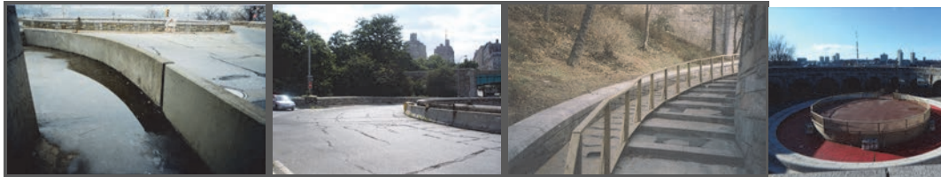
Traffic Circle Level: South Sidewalk Area - Extensive Water Ponding. Pavement - Widespread Cracking. Pedestrian Plaza Level: North Stairway - Timber Delivery Ramp. Closed Fountain.
