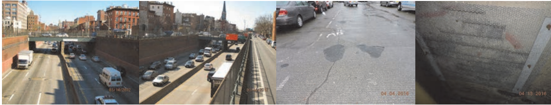
Sackett Street Bridge Over Brooklyn-Queens Expressway. March 2012: Elevation Left and Right. April 2016: Span 1 Wearing Surface. Span 2, Underside of Reinforced Concrete Deck Near the End Abutment - Exhibits a Spalled Area With Exposed and Corroded Rebars. This Location is Protected by Wire Mesh Netting. (Credit: NYSDOT)
