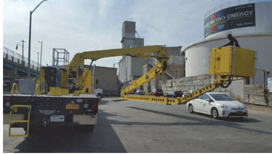
September 2017: Highway Repairer Dushawn Davis in the Bucket Practicing Deploying the Snooper Outside the Greenpoint Avenue Bridge Yard. (Credit: Mitul Patel)
