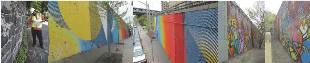
Inspecting a Bulge in a Retaining Wall Along Douglas Road in Staten Island in 2014. Brooklyn-Queens Expressway (BQE) Retaining Wall Between Washington and Adams Streets - Looking Northeast and Southwest. BQE Retaining Wall Between Adams and Pearl Streets - Looking Northeast and Southwest.
