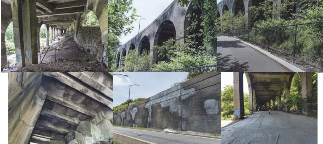
May 2017: Spans 36 to 25. Shotcrete Arch Repairs on Spans 34-32. Fence Restoration. Shotcrete Deck Repairs. Rebuilt Parapet.
