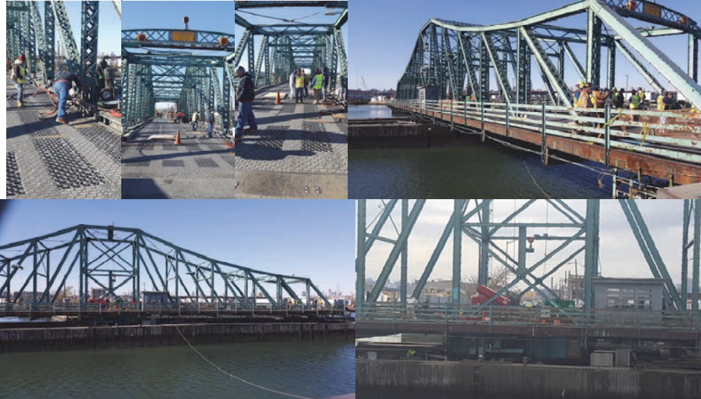
November 2017: Division Crews Addressed Multiple Red PIA Flags on the Grand Street Bridge. Work Included the Repair, Replacement, and Reinforcement of Stringers on Spans #1 and #2 as Well as Repairs to the Deck Grating and Roadway Plates. (Credit: Earlene Powell)
