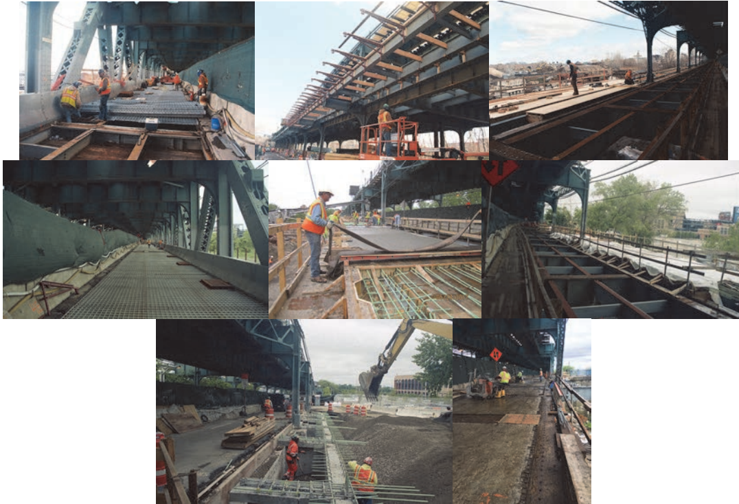
March 2017: Bascule Span - Installing Grid Deck for the Roadway. April 2017: West Viaduct – Formwork for the North Sidewalk. May 2017: Bascule Span Deck. West Viaduct – Stage 1 Sidewalk Test Panel Concrete Placement. West Approach – Stage 1 Sidewalk Preparation. East Viaduct – Stage 1 – Removing the Original Roadway Deck.
