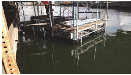
Inspector Utilizing a Motorized Platform Boat With Scaffolding to Access Most of the Underside of the Grand Street Bridge over Newtown Creek in November 2017. (Credit: NYS DOT)
