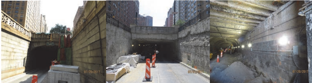
July 2017: Elevation South and North. South Portal Segment, Looking Northeast - Concrete Slab on Grade is Removed. Temporary Lighting Fixture Installed on the East Liner.
