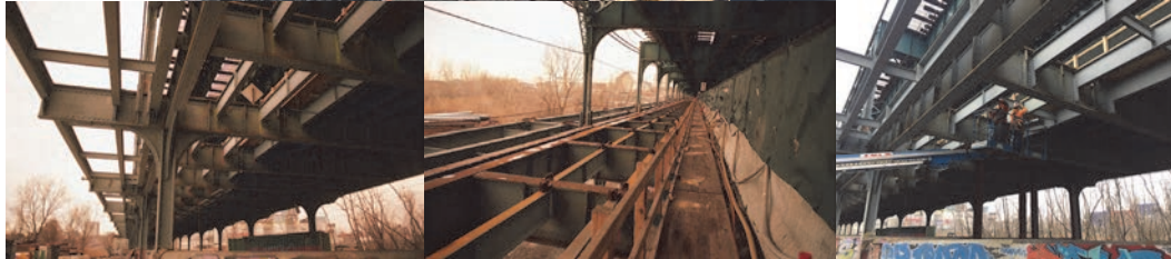
January 2017: Disconnecting the Existing Steel Grid Deck in the Bascule Span, Using a Torch, so That it can be Removed in Panel Sections. The Existing Grid Deck was Removed Entirely on the West Viaduct; the Existing Floor Beams Were Being Prepared for the Installation of New Stringers and Grid Deck Panels. On the Opposite Side of the NYC Transit Columns, New Sidewalk Steel was Being Installed. West Viaduct – Installation of Roadway Stringers for Stage 1. Inspecting the NYCT Columns and Removing Concrete Fill. February 2017: West Viaduct – Stage 1- Installing New Steel Under the Roadway Deck.
