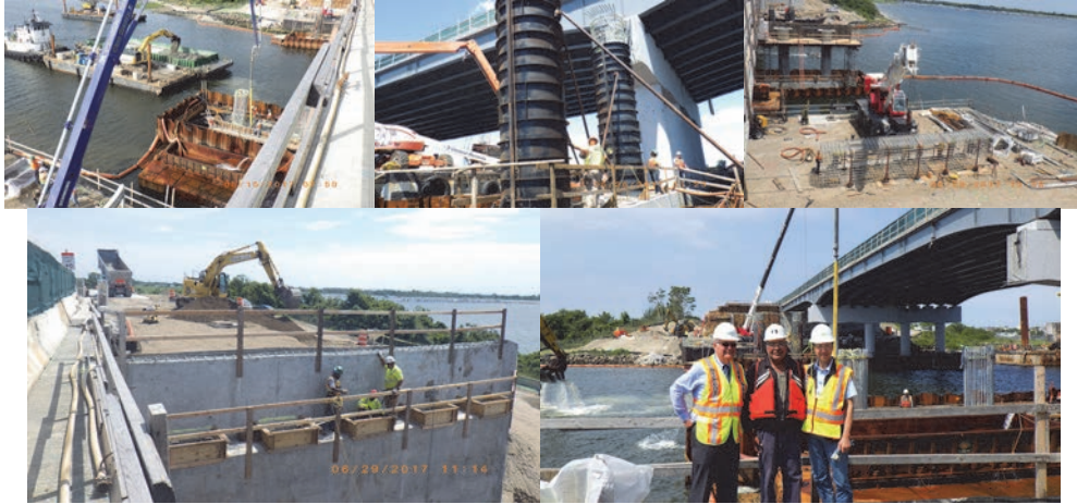
Gerritsen Inlet June 2017: Pumping Concrete for Plinth at Pier #2. Barge Mounted Backhoe Removing Blasted Concrete Debris From the Navigable Channel and Placing it on the Barge. Placing Reusable Column Forms on Top of Completed Plinth at Pier #2. Prefabricated Rebar Cage for Pier #1 Cap Beam to be Placed on Columns (Visible at Left) Completed Previously. Setting Forms for Bearing Pads at the East Abutment. Site Visit: Chief Bridge Officer Robert Collyer, Quality Assurance Assistant Civil Engineer Khalid Mohammed, and Administrative Engineer Daniel Hom.
