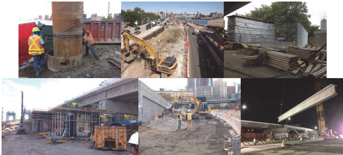
September 2017. October 2017: Enclosure to Protect the “Crack is Wack” Mural in the Park. Site View. Drainage Work at North Approach - Along Future Ramp D. November 2017: Last of the Pre-Stressed NEBT Girders for the Southbound Structure. (Credit: Artemio Angeles)
