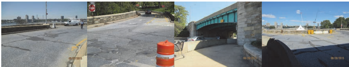
Traffic Circle Level – Spans 32, 14, and 15 Wearing Surface. (Credit: NYSDOT) Span 3, Traffic Signal at End-Center of Span.
