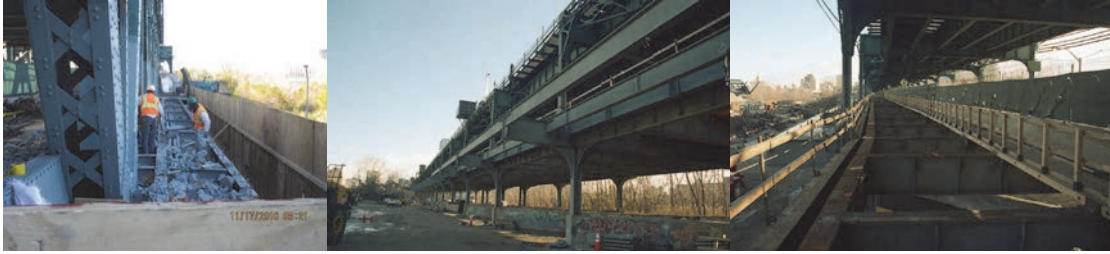
October 2016: Installing the New North Sidewalk – West Viaduct, Looking East. November 2016: Contractor Demolishes the Sidewalk over Van Wyck Expressway. East Viaduct – Stage 1 Installing the North Sidewalk Steel. December 2016: Installed North Sidewalk Stringers. West Viaduct – Roadway Deck Removed.
