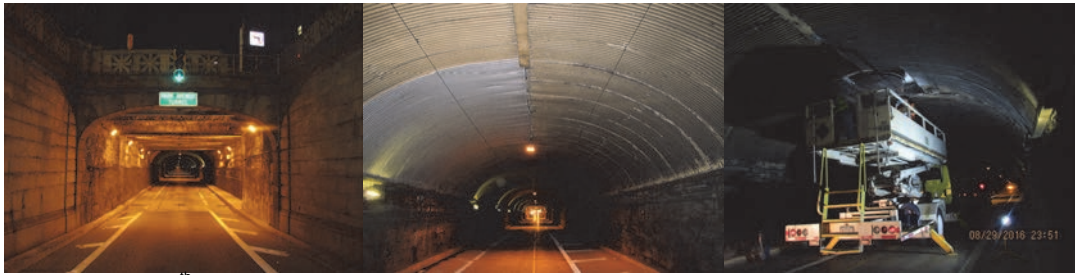
March 2016: 34 th Street Entrance, Looking Northeast. March 2016: Missing Joint Plates at Tunnel Crown. August 2016: Performing Overnight Preventive Maintenance.
