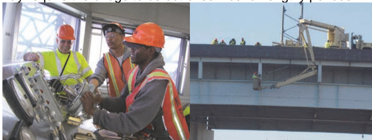
Construction Project Manager Gholamali Mozaffari, and Electricians Nelson Crooks and Gary Emmanuel Fixing Machinery in the Ninth Street Bridge Operator House in April 2008. (Credit: Vera Ovetskaya) Repairing the Navigation Lighting on the Hunterspoint Bridge. On the Bridge: Oilers Carl Wharton, Richard Morreale, and Paul Califano, Mozaffari Ali, Electrician Naum Golburt, and Highway Repairers Manny Nardiello and Kevin Donahue. In the Snooper Bucket: Harry Parmaman and Supervisor Electrician Jose Done. (Credit: Samuel Teaw)
