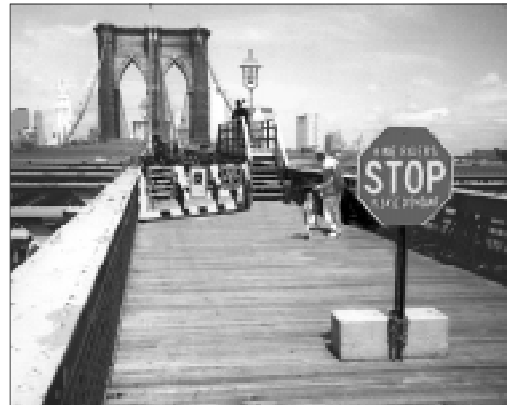
Temporary stair crossing over work zone during replacement of wood decking on the Brooklyn Bridge Promenade.
